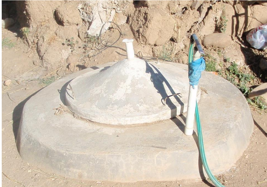
Figure 3-10. Surface view of EMAS underground tank with EMAS Pump
