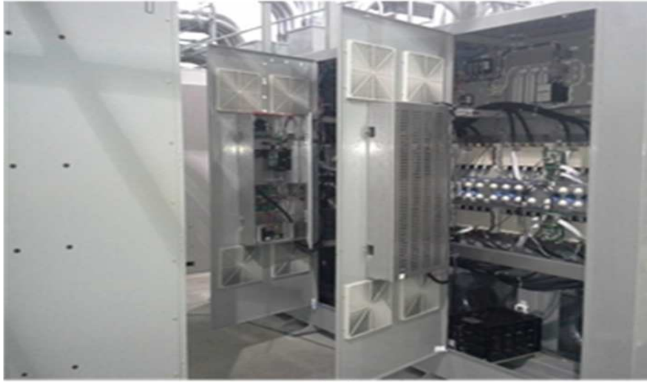
Figure B.7 DC Link Capacitors VVVF drive and REGEN Bench.
