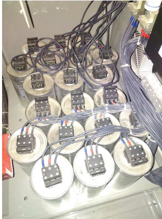
Figure B.4 Filter Capacitors in VVVF drive.
