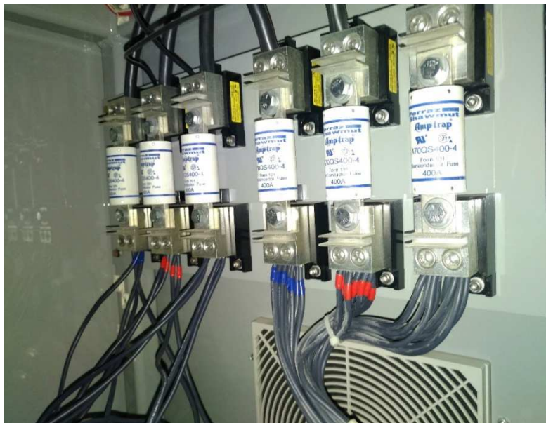
Figure B.5 Fuse Connection of Filter Capacitor for Rectifier and Inverter of VVVF.
