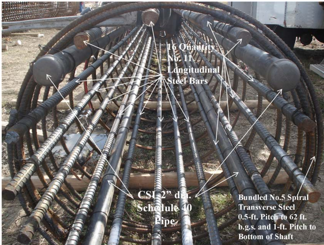
Figure 6.4. Photograph of an end view of the four-foot diameter shaft reinforcement cage.
