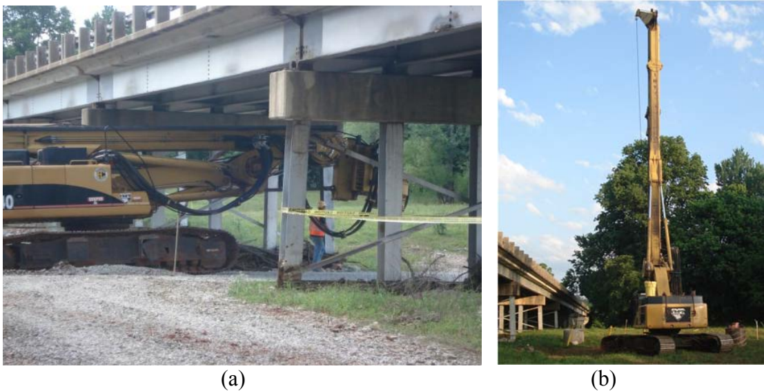
Figure 5.8. Photograph of Caterpillar AF 240 drill rig (a) mobilizing at the Siloam Springs site, and (b) in full operation at the Siloam Springs Site.
