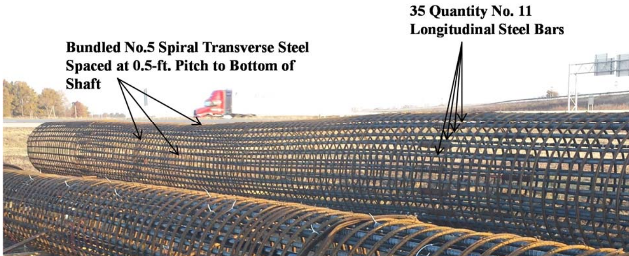
Figure 6.8. Photograph of a side view of the six-foot diameter shaft reinforcement cage.
