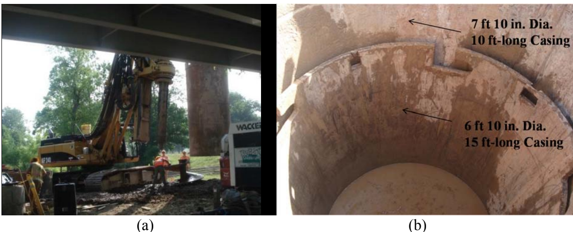
Figure 5.16. Photographs of Test Shaft SS-C6 (a) during the 15 foot length casing installation, and (b) after completed casing installation.
