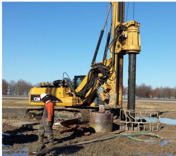
Figure 6.33. Photograph of the test shaft T-N4 excavation process utilizing the CZM I-25.
