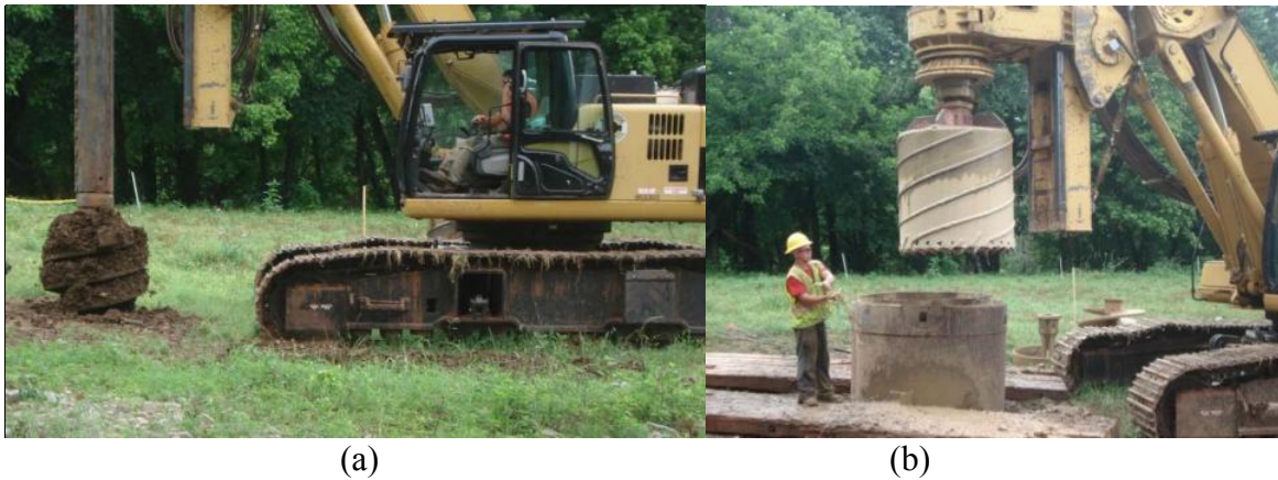
Figure 5.12. Photographs of Caterpillar AF-240 drill rig utilized to excavate Test Shaft SS-W4 with (a) a flight auger, and (b) a rock core barrel.
