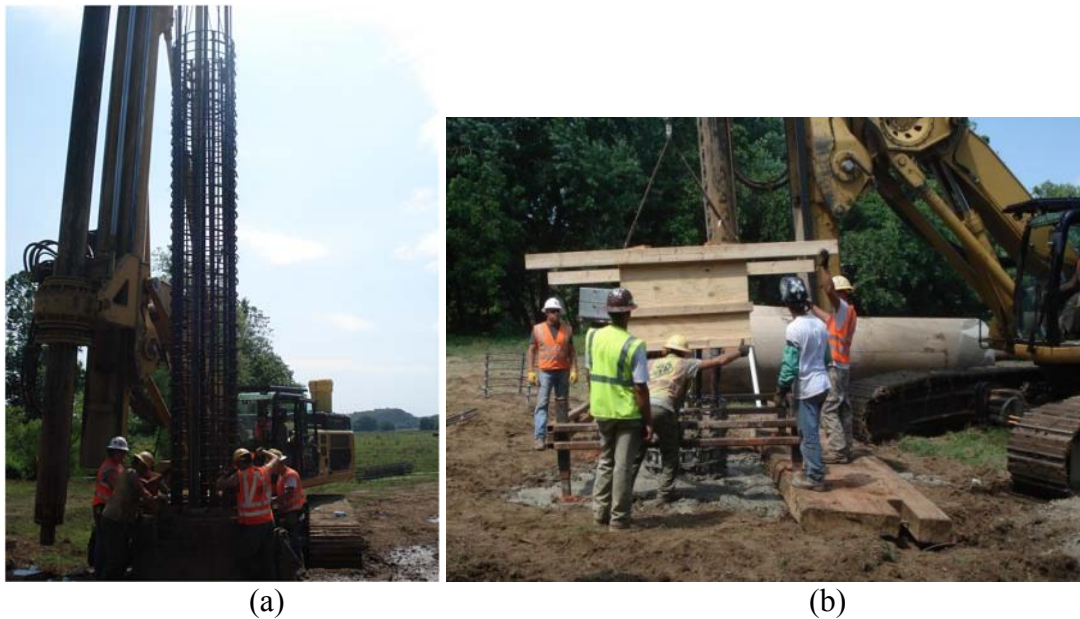
Figure 5.14. Photograph of Test Shaft SS-W4 (a) poured excavation casing removal and prior to placement of the square cap, and (b) three foot reveal placing form work for square cap.
