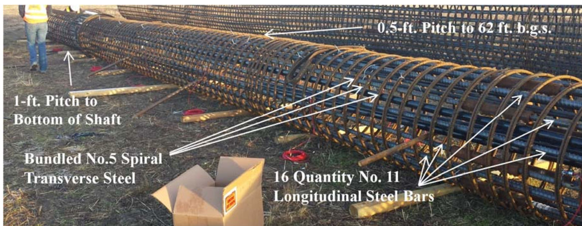
Figure 6.3. Photograph of a four-foot diameter shaft reinforcement cage from the side view.
