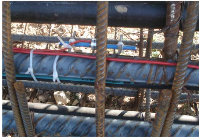
Figure 5.7. Photograph of installed vibrating wire strain gauge utilizing welded mount and zip ties.
