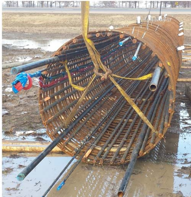
Figure 6.27. Schematic of (a) top-down view of test shaft T-C6, and (b) photograph of instrumented assembly.
