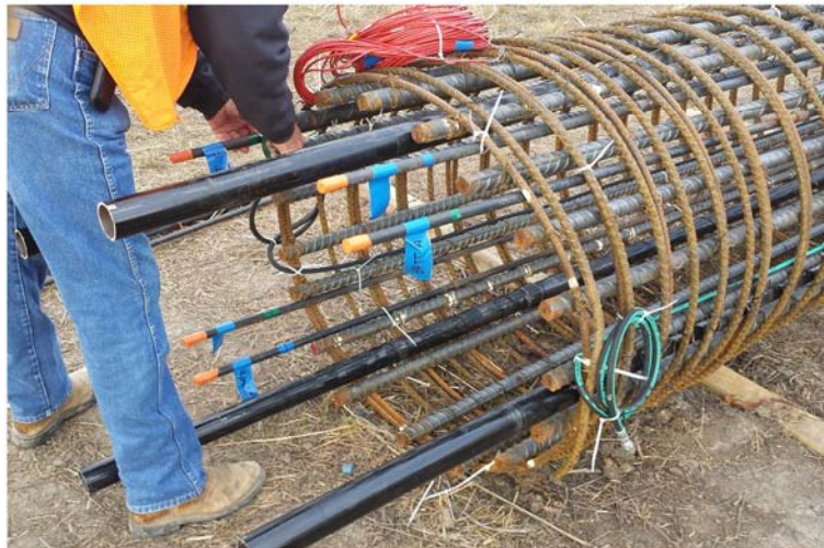
Figure 6.23. Schematic of (a) top-down view of test shaft T-4S, and (b) photograph of instrumented assembly.
