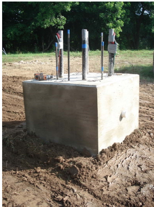
Figure 5.15. Photographs of Test Shaft SS-W4 (a) rebar cage, and (b) finished construction.
