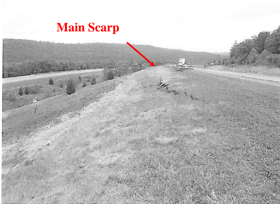
Figure 3.3. Looking north to the main scarp at the calibration site near Chester, Arkansas in May 2010 (from AHTD, 2010).
