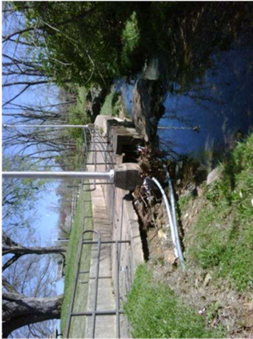
Figure 16a. Sidewalk area prior to 2009 repairs
