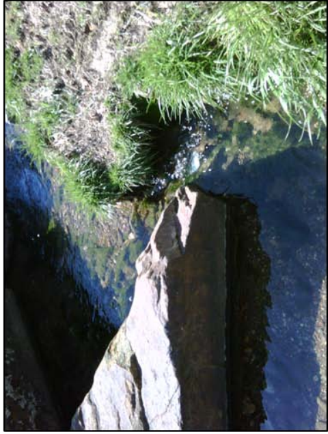
Figure 4c. Misplaced boulder causing flow diversion and erosion
