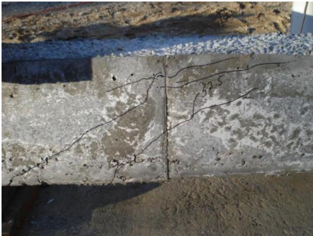
Figure 6.11: Shear cracking of specimen NSC-3L
