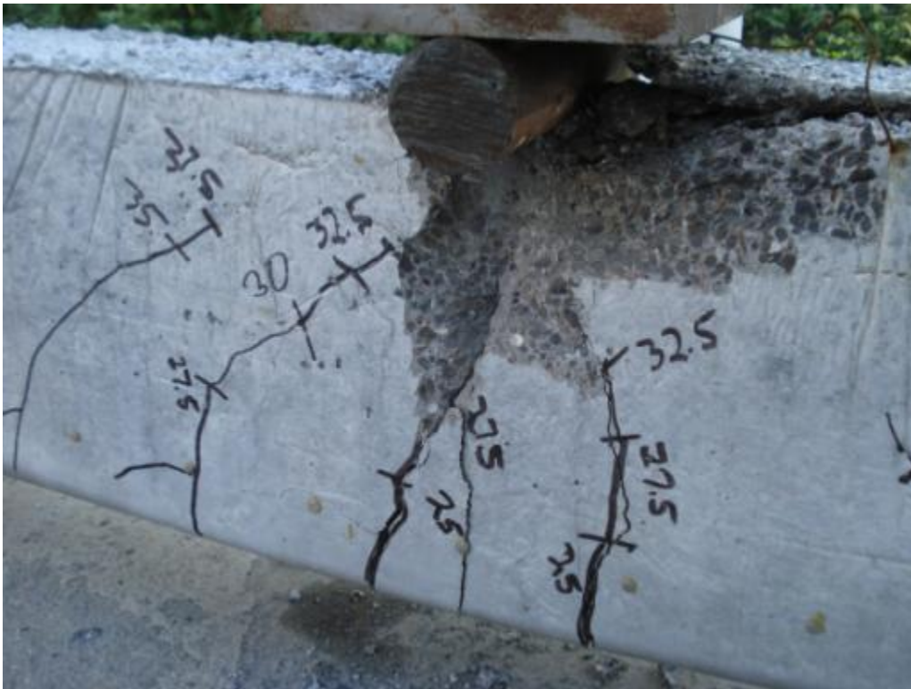
Figure 6.30: Failure of specimen NSS-4D
