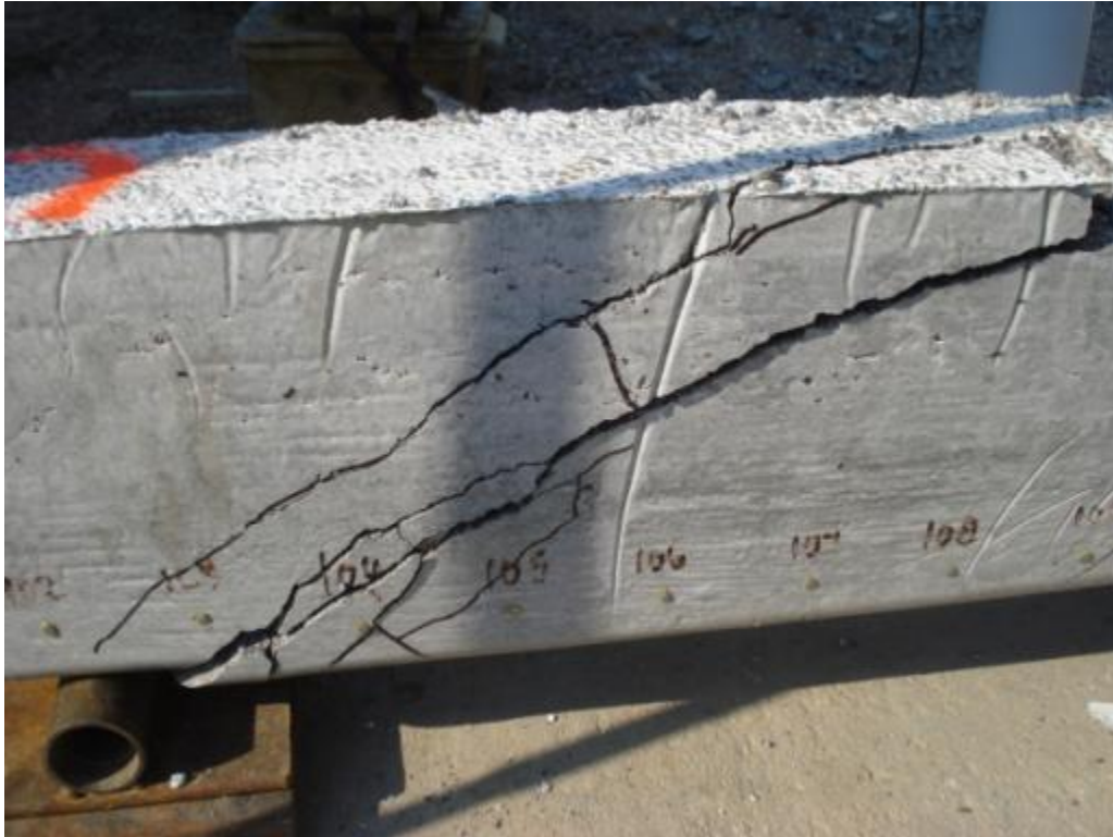
Figure 6.32: South side shear cracking of specimen NSS-4L
