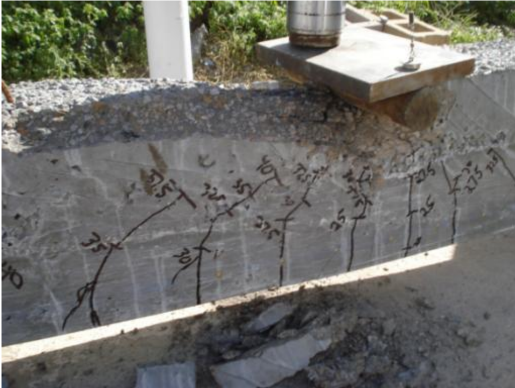
Figure 6.67: Cracking and failure of specimen HSC-4L
