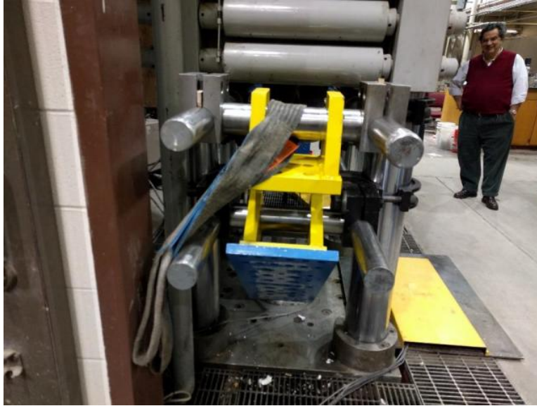
Figure 13 – With reaction bars in place, rod clamps and clevis brackets are installed.
