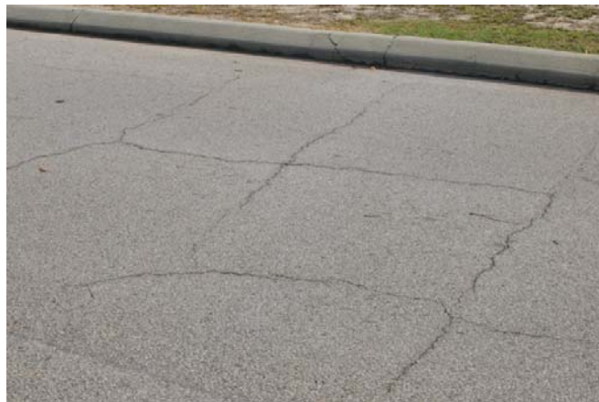
Figure 2.4: Pattern cracking of concrete pavement (LGAM, 2011)
