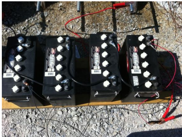
Figure 4.1: Deep cell batteries (Osweiler, 2012)
