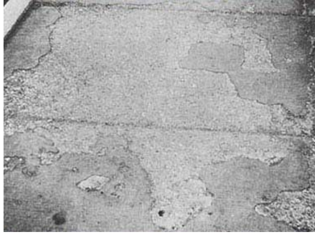
Figure 2.3: Scaling of aggregate (Concrete Ideas, 2011)
