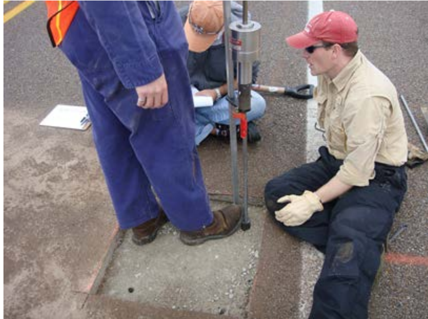
Figure 6.5. DCP test conducted in southeast corner of excavation area of Section 13W.
