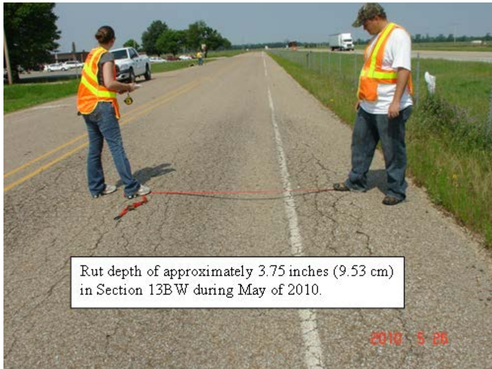
Figure 6.1. Rut depth exceeding 3 inches (7.6 cm) in Section 13BW during May 2010.
