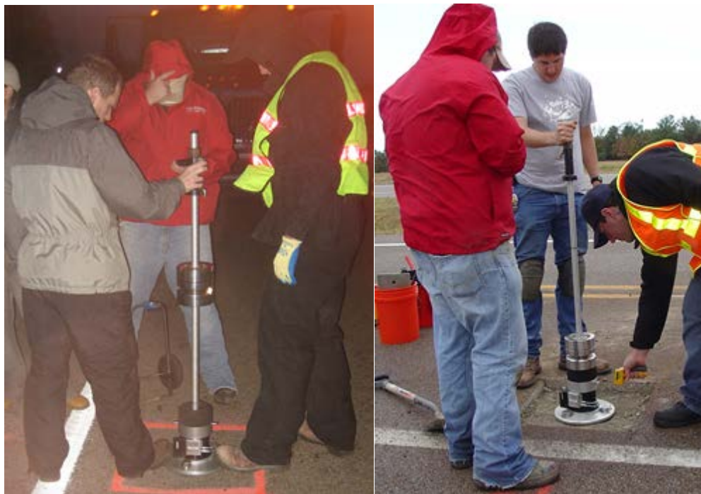
Figure 5.19. LWD tests conducted on asphalt and base course layers at Marked Tree site.
