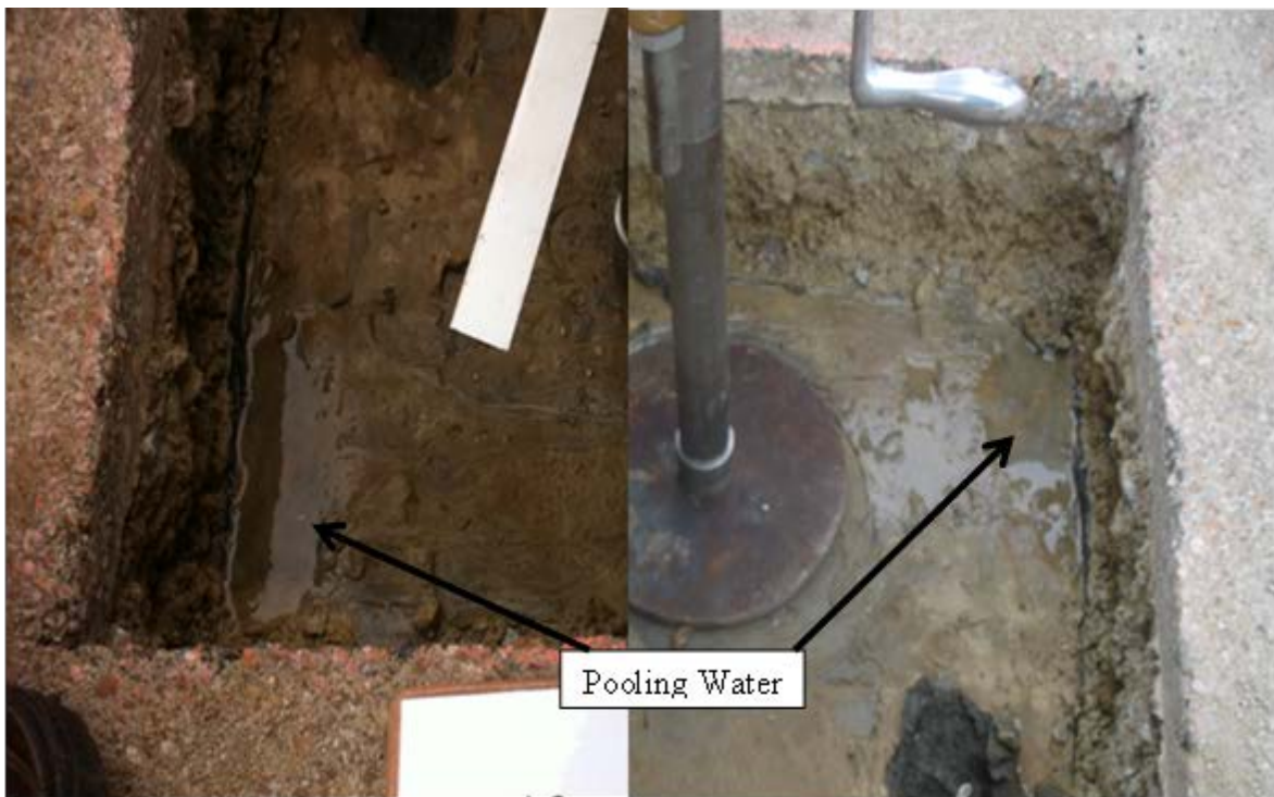
Figure 6.15. Pooling water on subgrade of Section 13W in October 2010.
