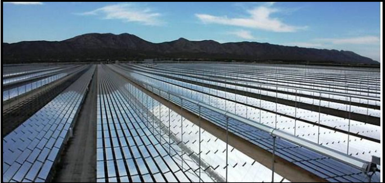
Figure 4: Linear Fresnel Array at the 30 MW Puerto Errado 2 CSP Plant in Calasparra, Spain (PE2, 2010)
