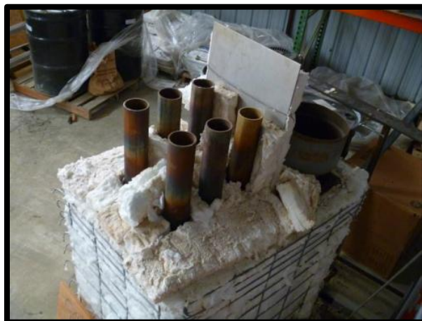
Figure 50: Insulated Salt Storage Tank
