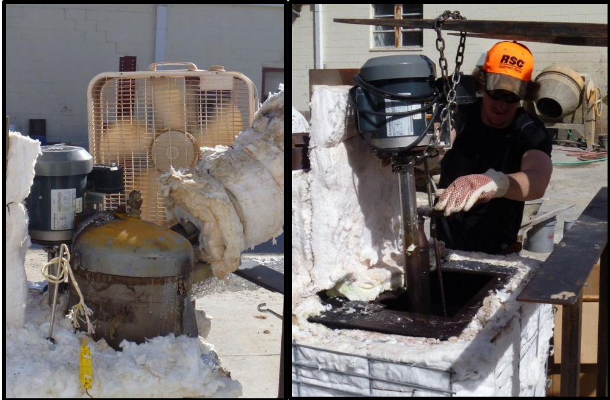
Figure 69: Motor Driving Pumping Unit During Testing (Left) and Pumping Unit Being Removed to Allow Replacement of First Motor (Right)
