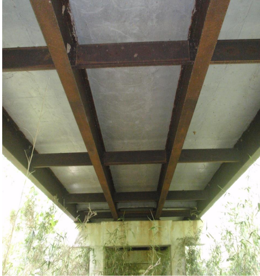
Figure 4.2: Hartbarger Bridge – view of framing plan from underside of bridge. Photo taken by Jeremy Rawn, Fall 2010 Fayetteville, Arkansas
