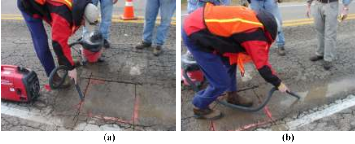
Figure 3.4. Water introduced by cutting the asphalt removed by a portable vacuum a) within the test section and b) around the test section.
