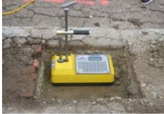
Figure 3.15. Nuclear gauge positioned to obtain subgrade density and water content readings (Section13BW).
