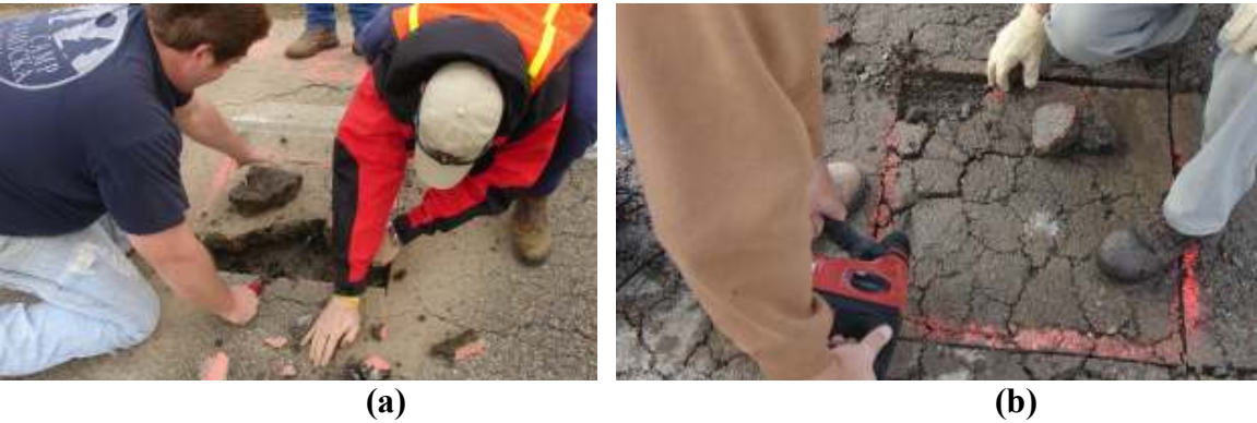
Figure 3.5. Removal of asphalt using a) crowbar (Section 13W) and b) hammer drill (Section 13BW).
