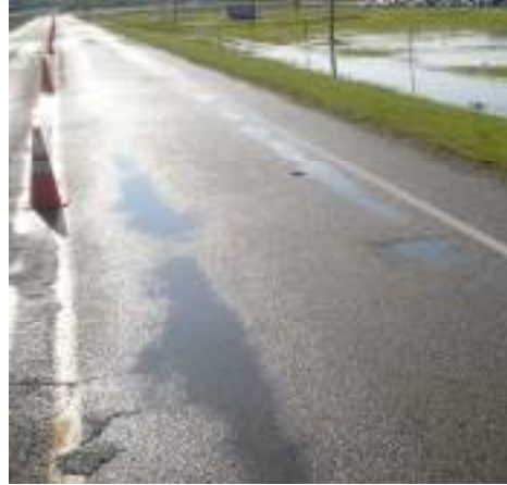
Figure 4.37. Ponding in six-inch thick sections in May, 2011 (from Goldman, 2011) [view from Section 13W looking East].
