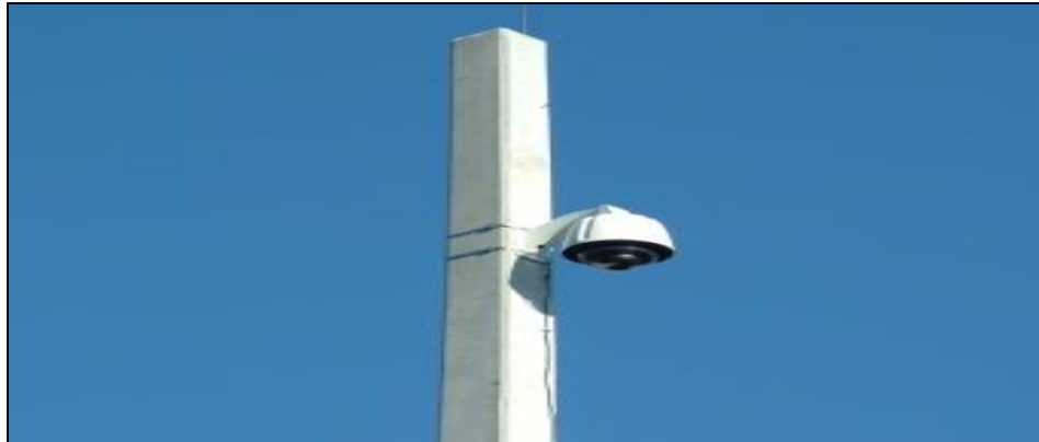
Figure 4.3 Closed Circuit Television Camera
