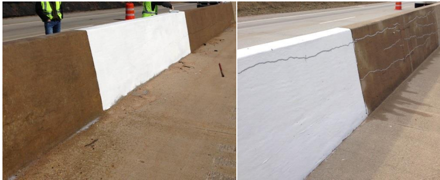
Figure 2.10. Application of surface treatment (left) and crack sealant (right). Pictures used with permission from Richard Deschenes.
