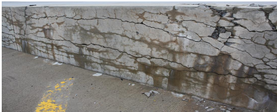
Figure 2.3. A typical median barrier section which exhibits severe damage, (e.g. severe map cracking, longitudinal cracks, crushing at the joints, and visible alkali-silica gel exudation). Picture used with permission from Richard Deschenes.
