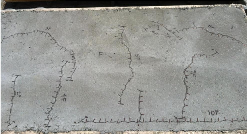
Figure 4.14 Slab Cracks Mapped 24 Hours After Casting
