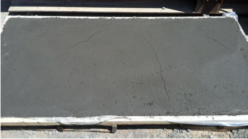
Figure 4.13 Slab After Formation of Plastic Shrinkage Cracks
