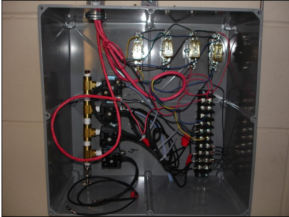
Figure 17: Image of the high-pressure pneumatic junction box.
