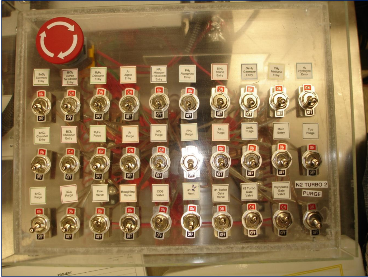
Figure 8: Photograph of main switchbox layout.
