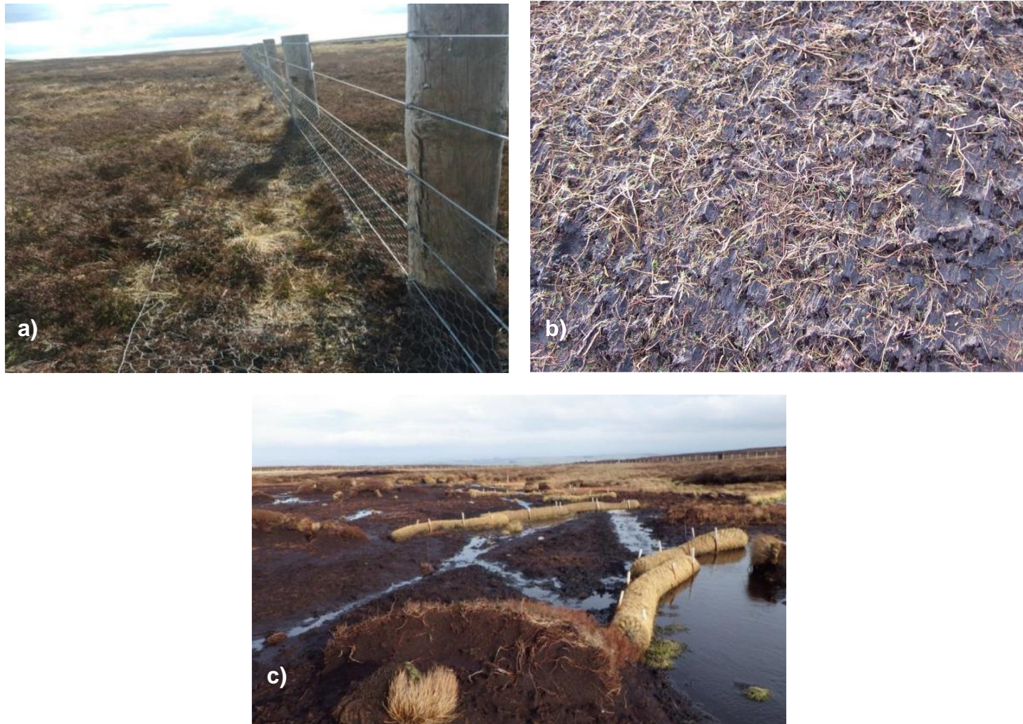
Figure 3.4 - (a) Sheep and rabbit fencing added in 2010, (b) heather brush spread to reduce bare peat erosion in November and December 2010, (c) Coir rolls to reduce surface erosion, added February 2013.
