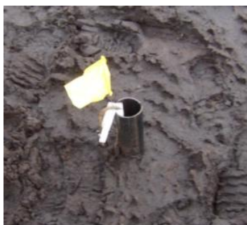
Figure 3.13: The Automatic Pressure Transducer installed in a well to measure the hydrological response of the blanket peat.
