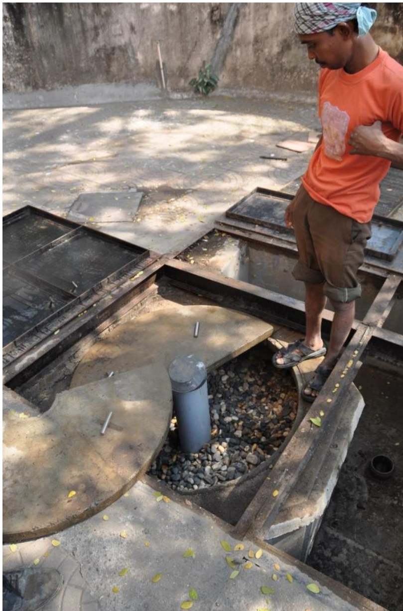
Figure 6.10: The gravel filters must be cleaned annually (Source: Author)
