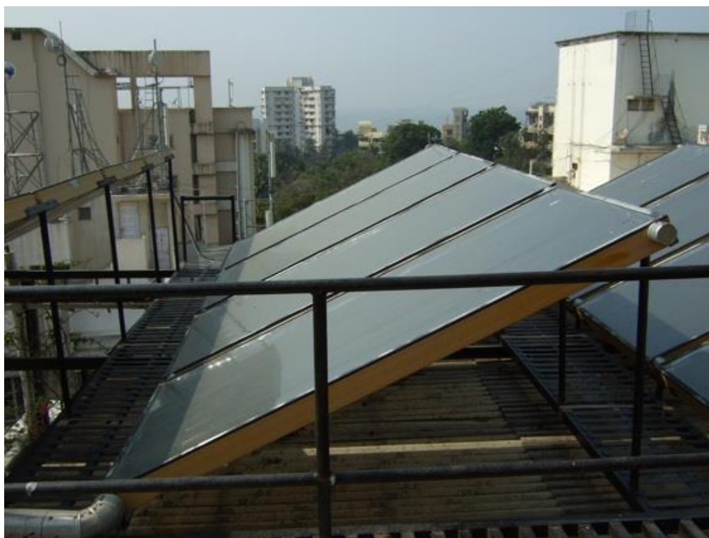
Figure 6.13: Solar water heating was installed after rainwater harvesting in Sealine (Source: Author)
