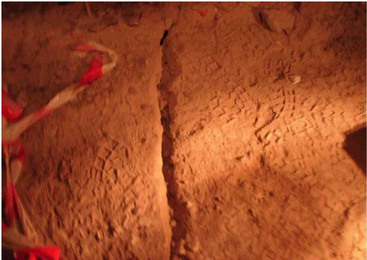
Plate 5.4 Crack on the floor across the roadway at site 2
