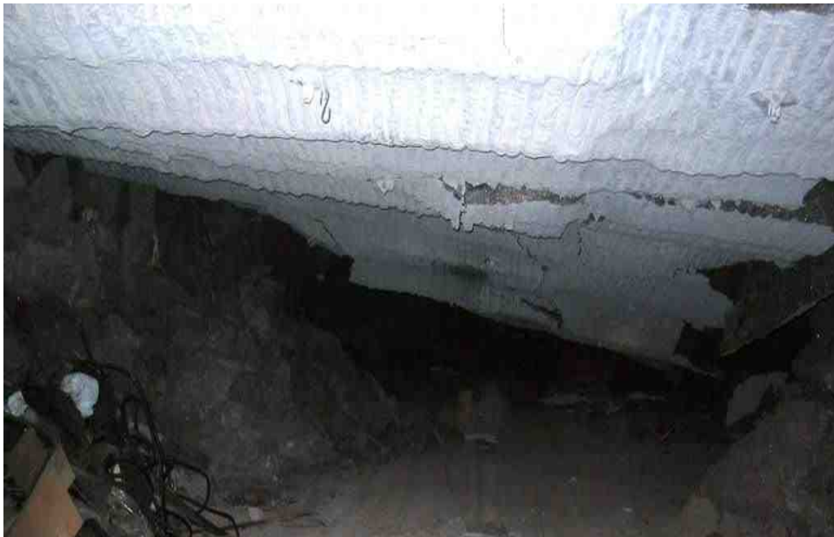
Plate 3.2 Closure in the underground working of Boulby mine in 2007. The roof has closed from over 3 m to less than 1.5 m in the foreground and almost completely in the background.
