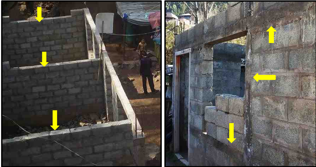
Figure 7.1 (left) An under-construction pukka house in rural Bagh with no plinth and lintel level beams in walls (yellow arrows) in contravention to the ERRA specifications; (right) a seismically compliant under-construction pukka house in rural Muzaffarabad with proper pillars and beams. (Source: Author fieldwork)
