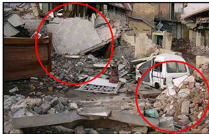
Figure 5.11 A pukka building in urban Bagh, mixed construction material (stones and bricks) is used in the same wall (picture above); destroyed pukka construction in urban Muzaffarabad, mixed construction material such as bricks and concrete blocks can be noticed in red circles (picture below). (Source: SERRA)
