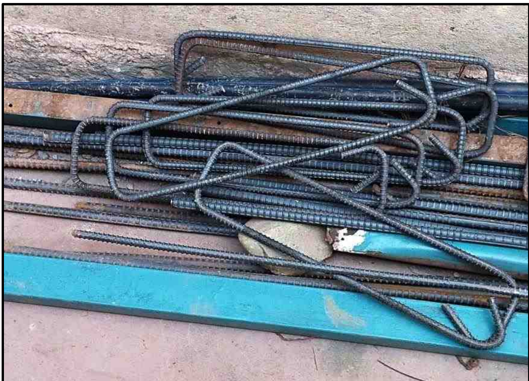
Figure 7.3 Properly formed steel rings for RCC frame structure, a rarity before the earthquake. (Source: Author fieldwork)
