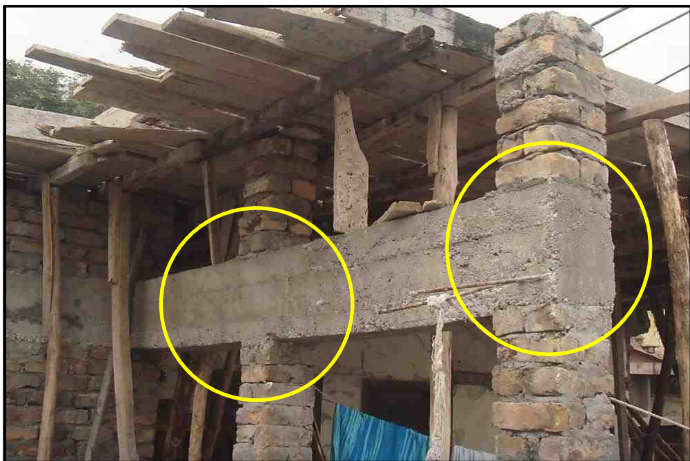
Figure 7.2 An under-construction house in Muzaffarabad city; notice brick columns and concrete beam in utter violation of the engineering principles (yellow circles). (Courtesy: Sheikh Ahsan)
