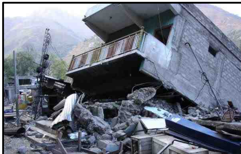
Figure 5.12 A Destroyed Pakka House
