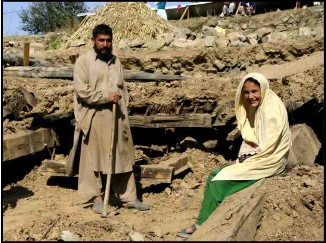
Figure 5.8 A destroyed Kacha house: note heavy wooden beams, loose joints, undressed stones and thick mud roof. (Source: ERRA 2015)
