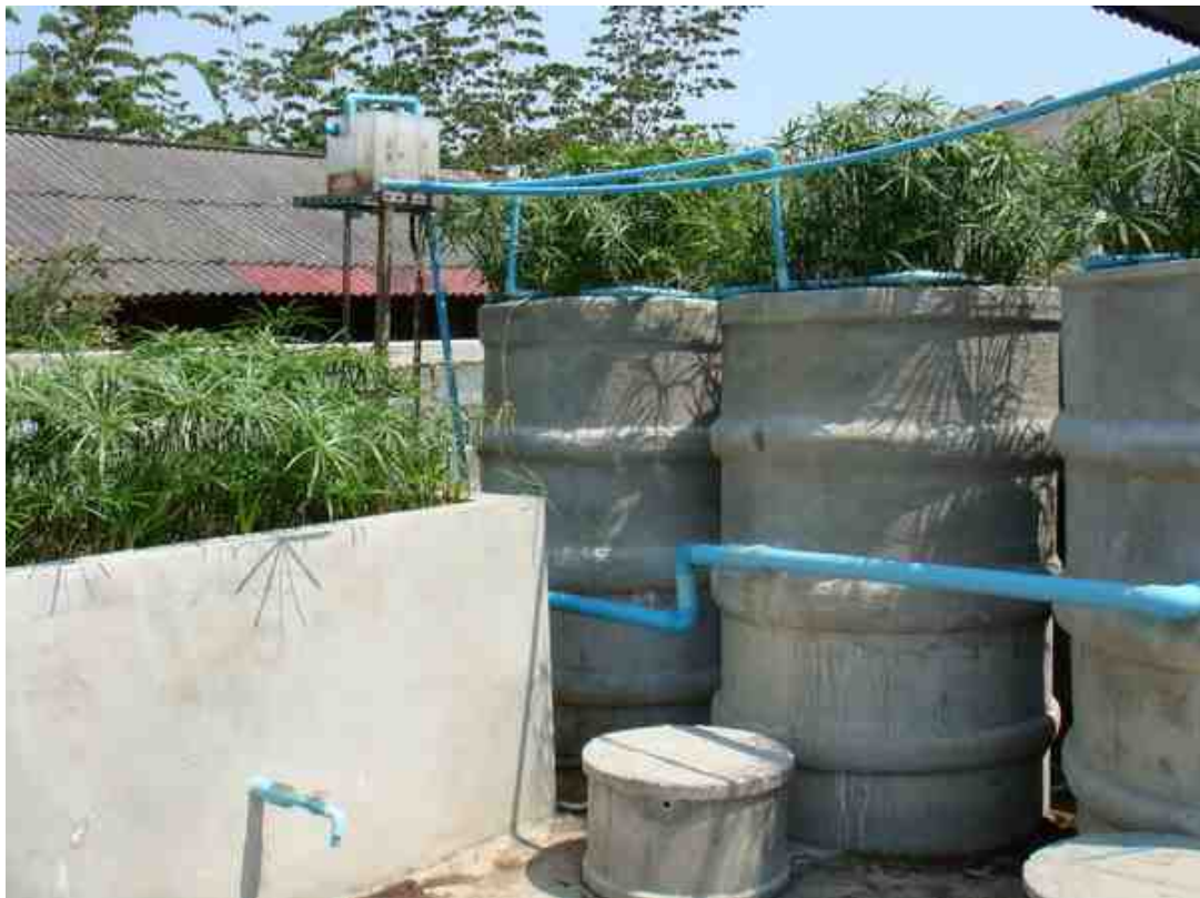
Picture 6.1 A Waste Water Treatment System, Baan Ton Pao
