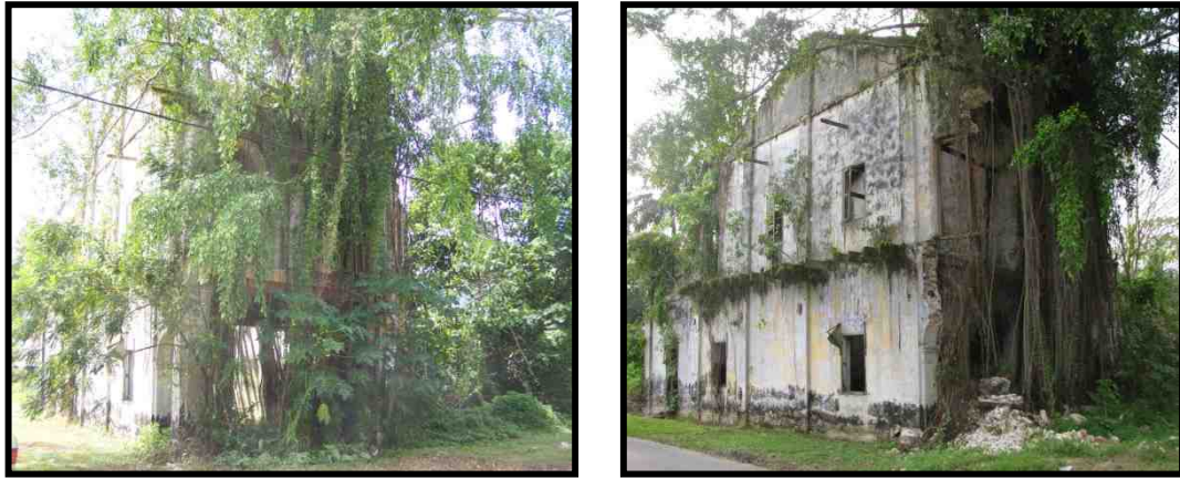
Fig. 1.4: Dilapidated buildings at Papan earning it a ‘ghost town’ status (source: author)
