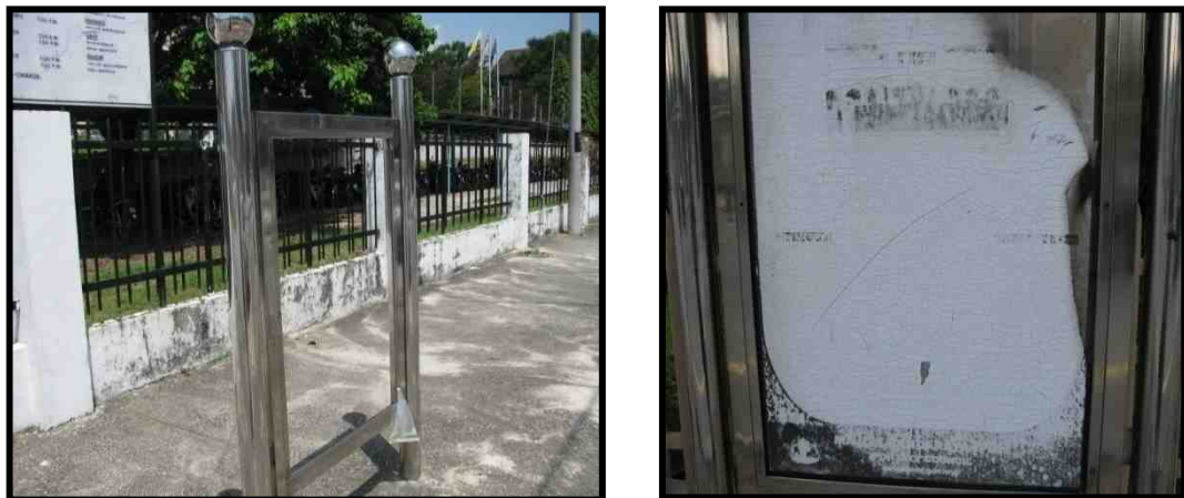
Fig. 5.20: Poorly maintained storyboards in Ipoh (source: author)
