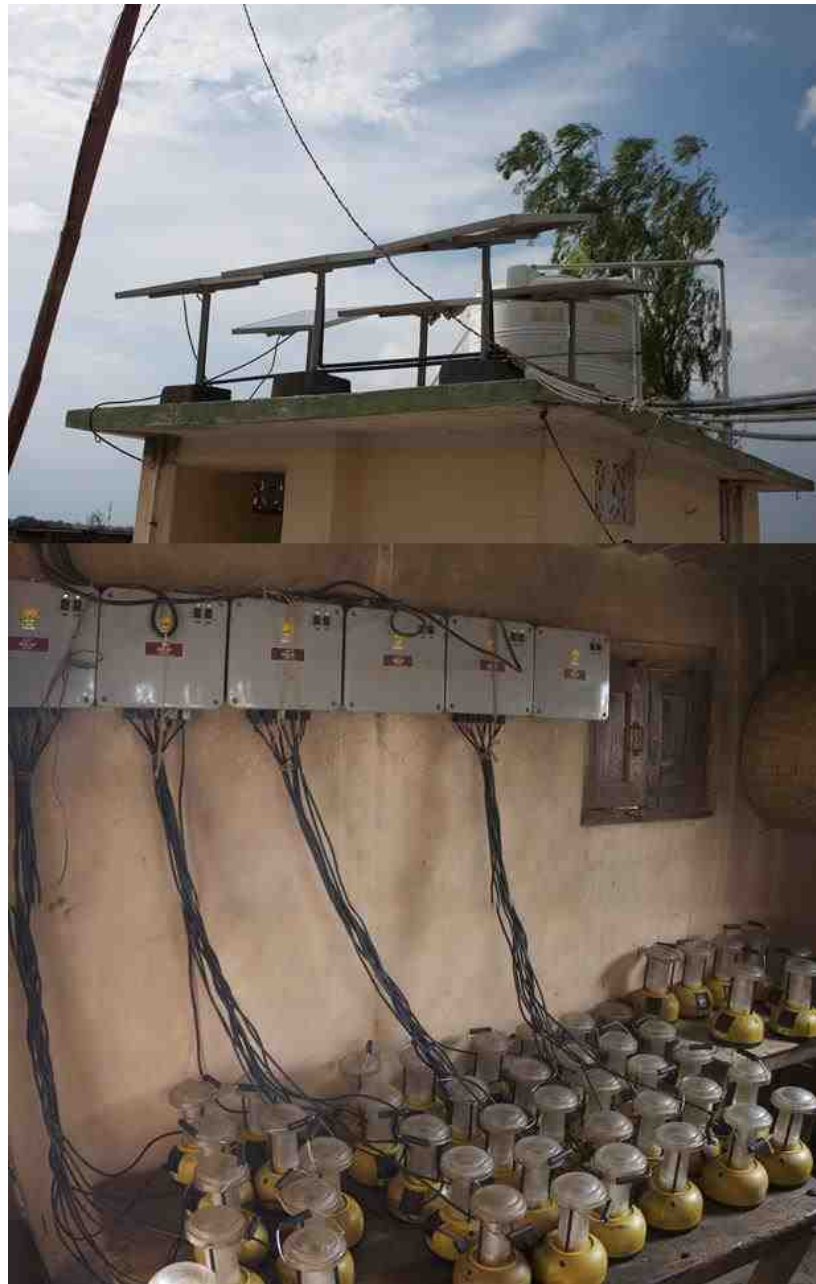
Figure 4-1: Solar panels (top) with charging station and solar lanterns (bottom).
