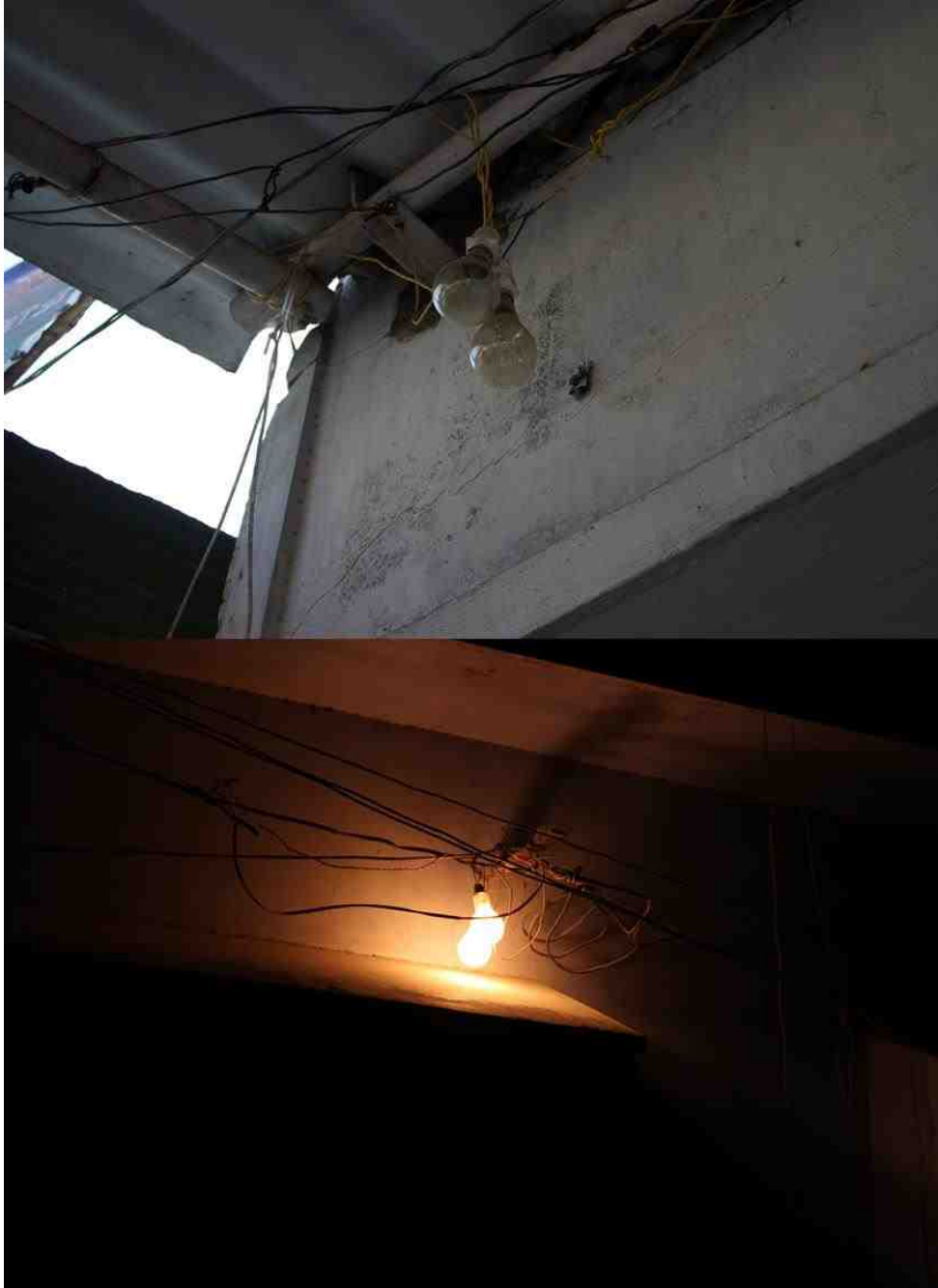
Figure 7-7: Bulbs used as 'choke points' by HPS.
