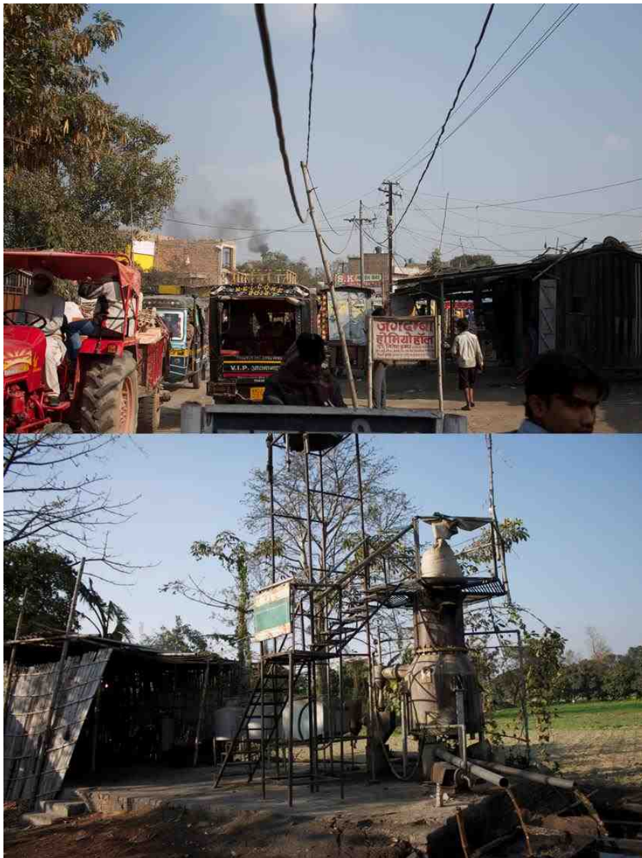
Figure 4-3: HPS gasification plant (bottom) and transmission lines (top).
