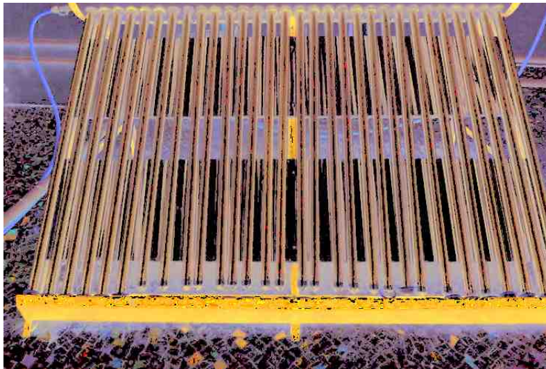
Figure 7.10: Malfunctioning SHW systems in social housing, Thane.
