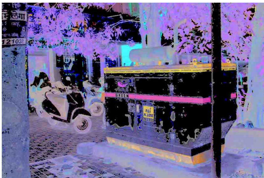
Figure 2.3: Private diesel generator for electricity provision, Thane.
