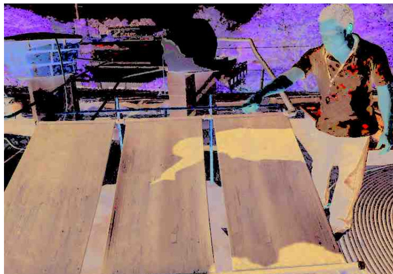
Figure 6.10: DIY SHW system installed at the roof of offices of the Sociedade do Sol , in São Paulo.
