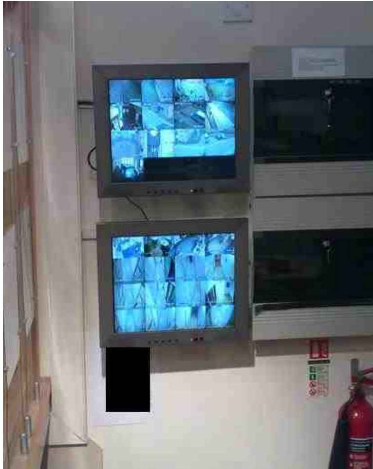
Figure 10 CCTV system at BP
