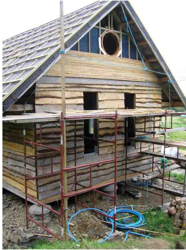
Figure 23: Outside of the barn showing the scaffolding used to work on, and my lathing contribution: the thin wood strips under the circular window (photograph: authors own)
