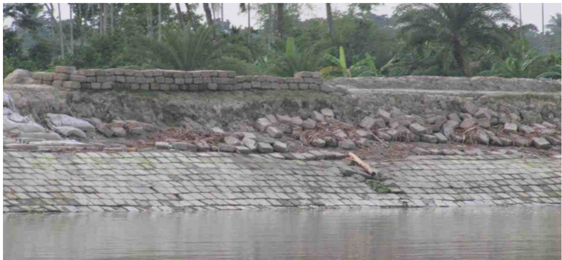
Figure 4.2: A damaged and poorly maintained part of embankment in the Sarankhola Upazila
