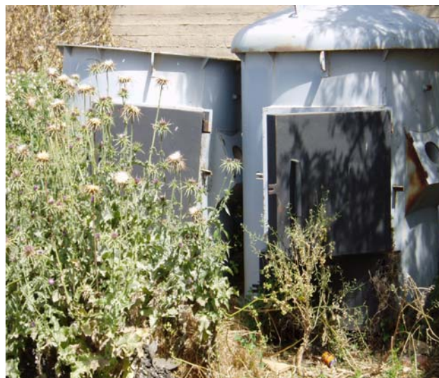
Fig. (18): Unused incinerator (Italian Donation) in the field near the waste water treatment plant in Jenin city 2007 (M .Abu Sroor 2007/4).
