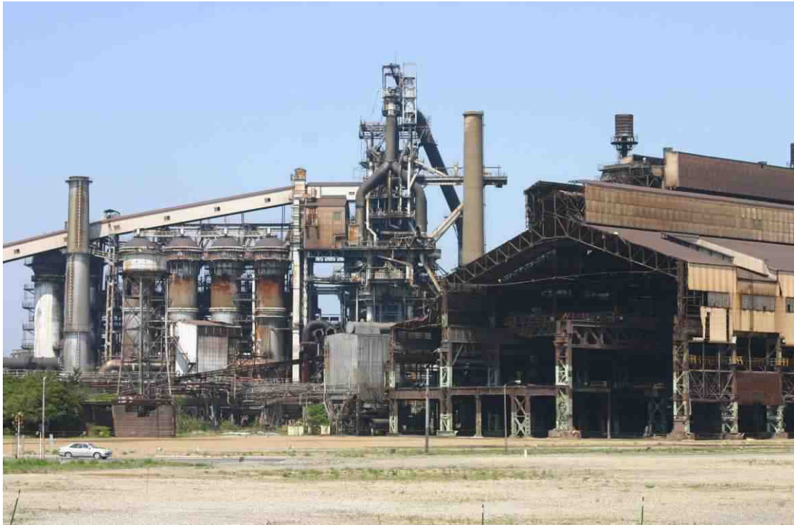
Fig.9.1: A changing order. In 2005 the first blast furnace and strip mill built in 1953 by Nishiyama Yataro are demolished in favour of a retail mall and a business innovation park.
