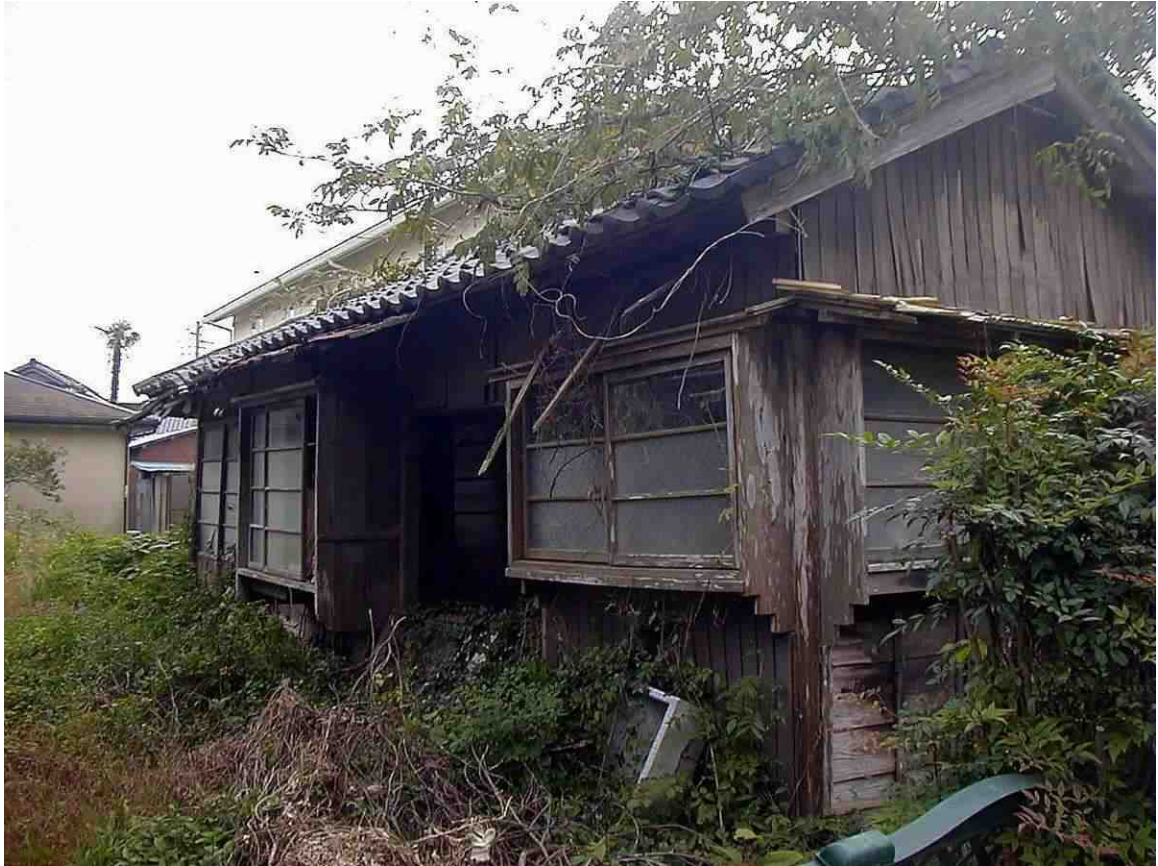
Fig.2.1:Redundancy and processes of physical decay. In the humid Kanto climate unmaintained and vacant wooden structures deteriorate within three to five years. Naruto-machi, Sanmu-shi .
