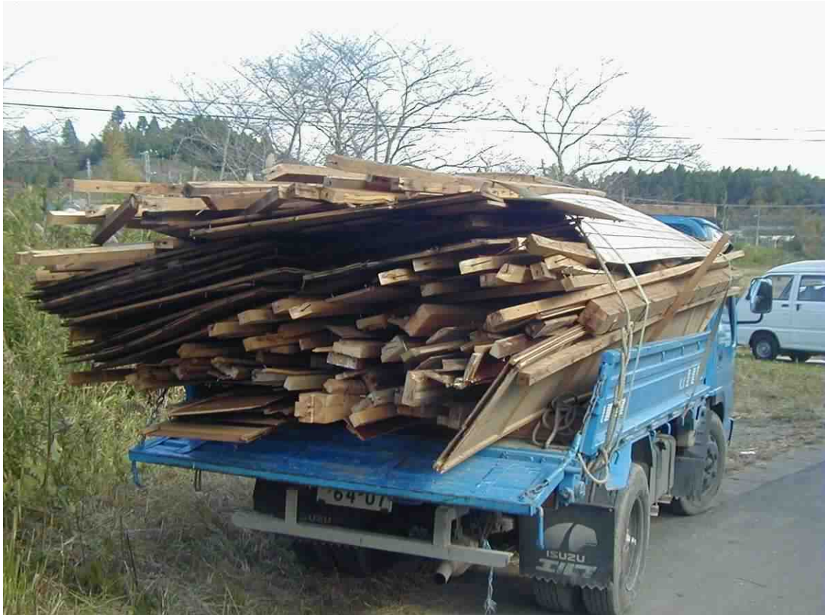
Fig.2.6: Taxonomy of change: qualitative change by substitution. It takes two men about three days to demolish an early 1960's wooden dwelling and leave a new building plot. Sammu-shi
