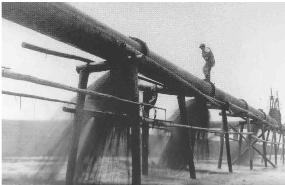
Fig. 7.2 'Dredge Reclamation' in progress on the foreshore at Inage 1964. This was the commonest technique used for landfill and consists of pumping silt dredged offshore into banded areas as slurry and allowing the material to dry out and solidify into new ground.
