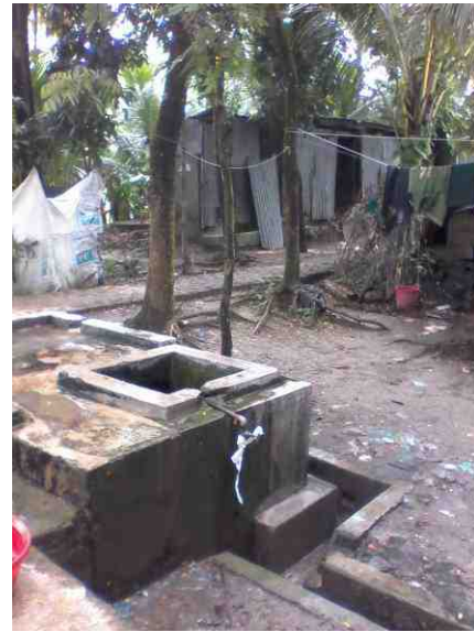
Tap water supply and sanitation system in a residential project of Government for the landless people
