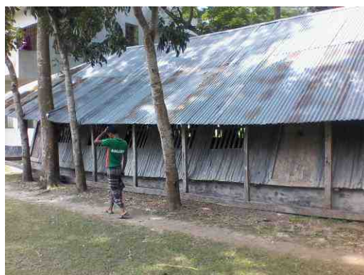
A school house damaged by the recent cyclone Mahasen in 2013
