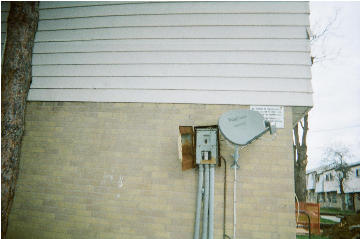
William’s photograph of an ill-maintained electricity meter box.
