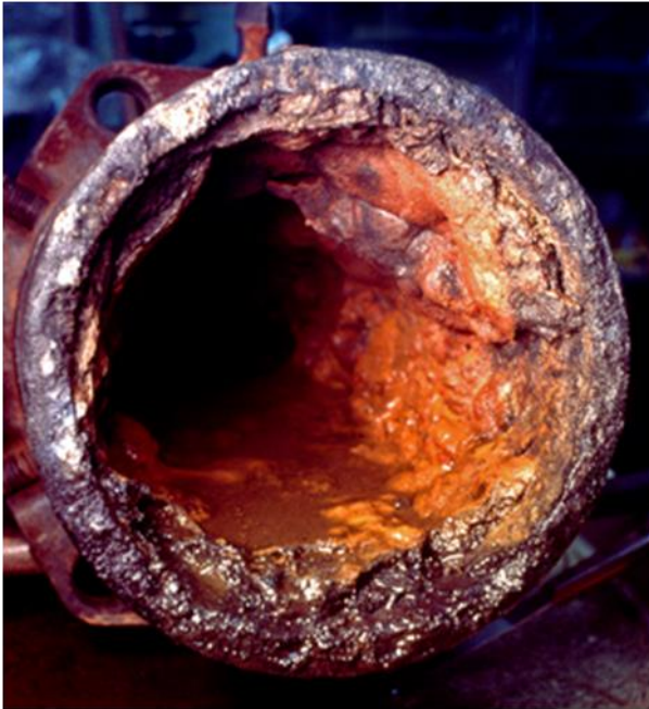
Figure 3. Biofilm growth in a drinking water supply pipe (ProEconomy 2015)
