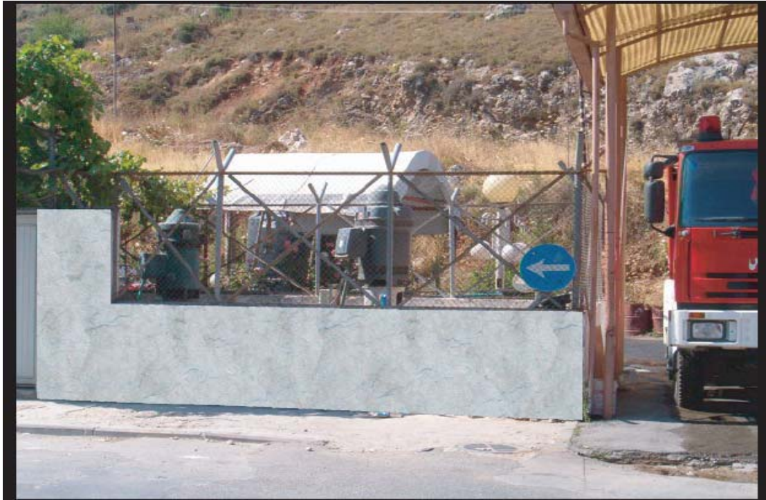
Alsumara Pumping Station
