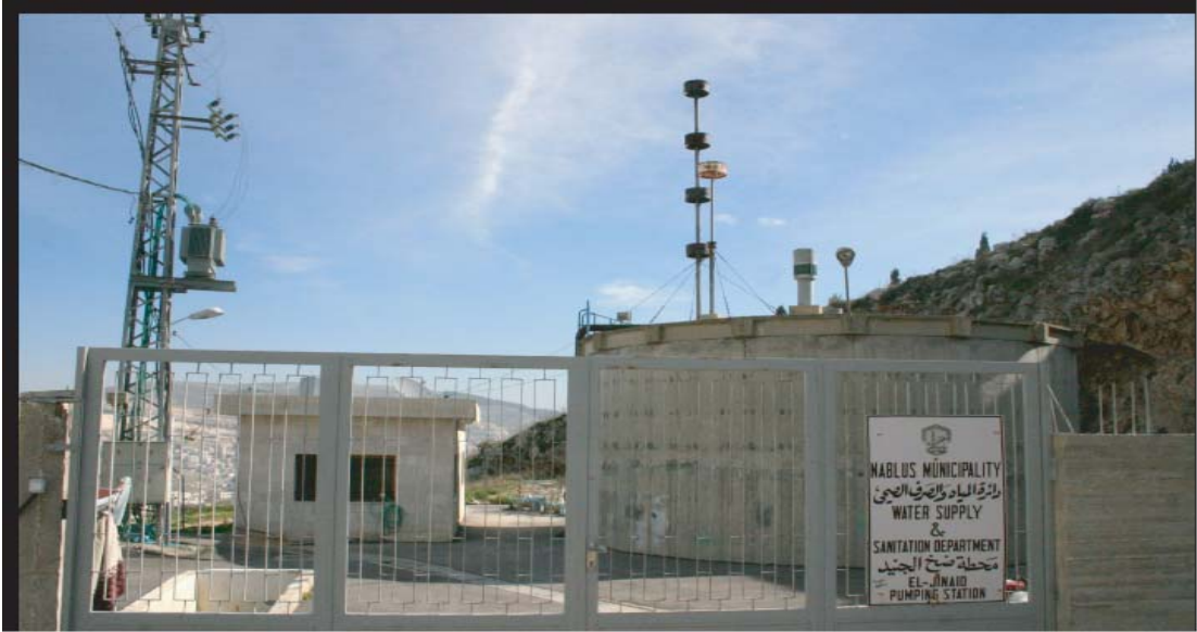
Aljunied Pumping Station
