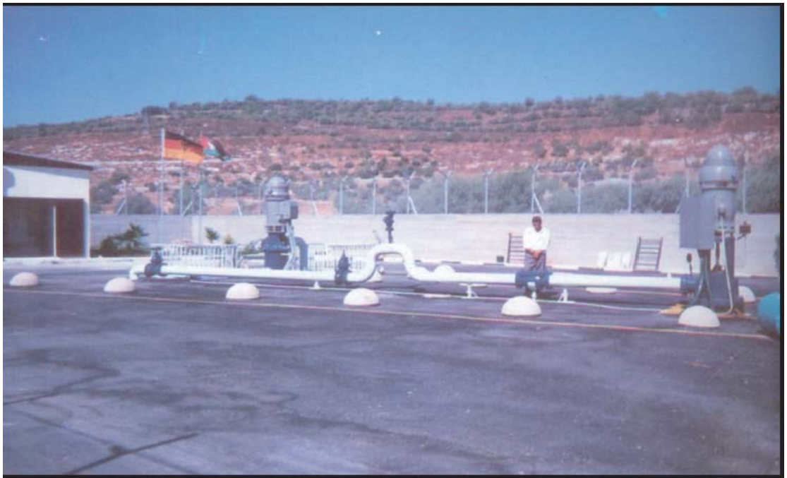
Deir Sharaf Pumping station
