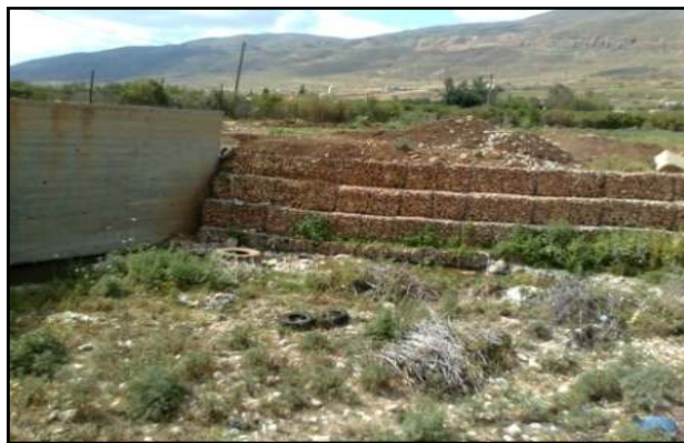
Figure (5.5): Side Armoring by Gabions used at Reach 4-5 of Faria Stream ( Near Aqrabania Entrance)
