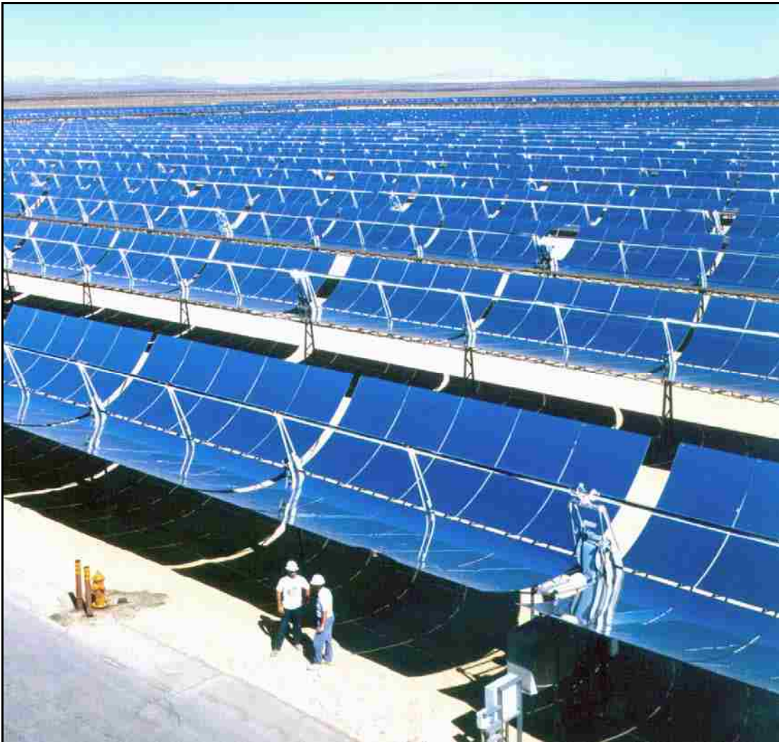
Figure 2. Parabolic Trough Mirrors at the SEGS IV CSP Facility in Kramer Junction, CA.
