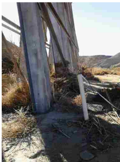
Figure 145. An Aligned PVC Pipe and the Adjacent Pile
