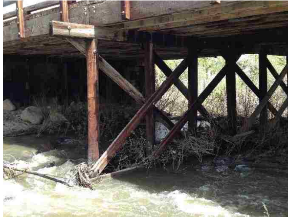
Figure 93. Street View of Bridge No. 1190 Showing Running Water Surrounding Intermediate Bent during the First Visit
