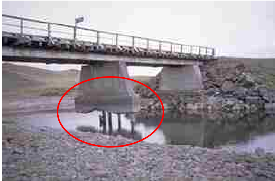
Figure 2. Complete Loss of Support under a Bridge Pier (3)
