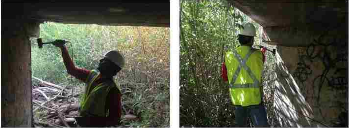
Figure 135. Upward Striking on the Pile Cap and on the Bridge Deck
