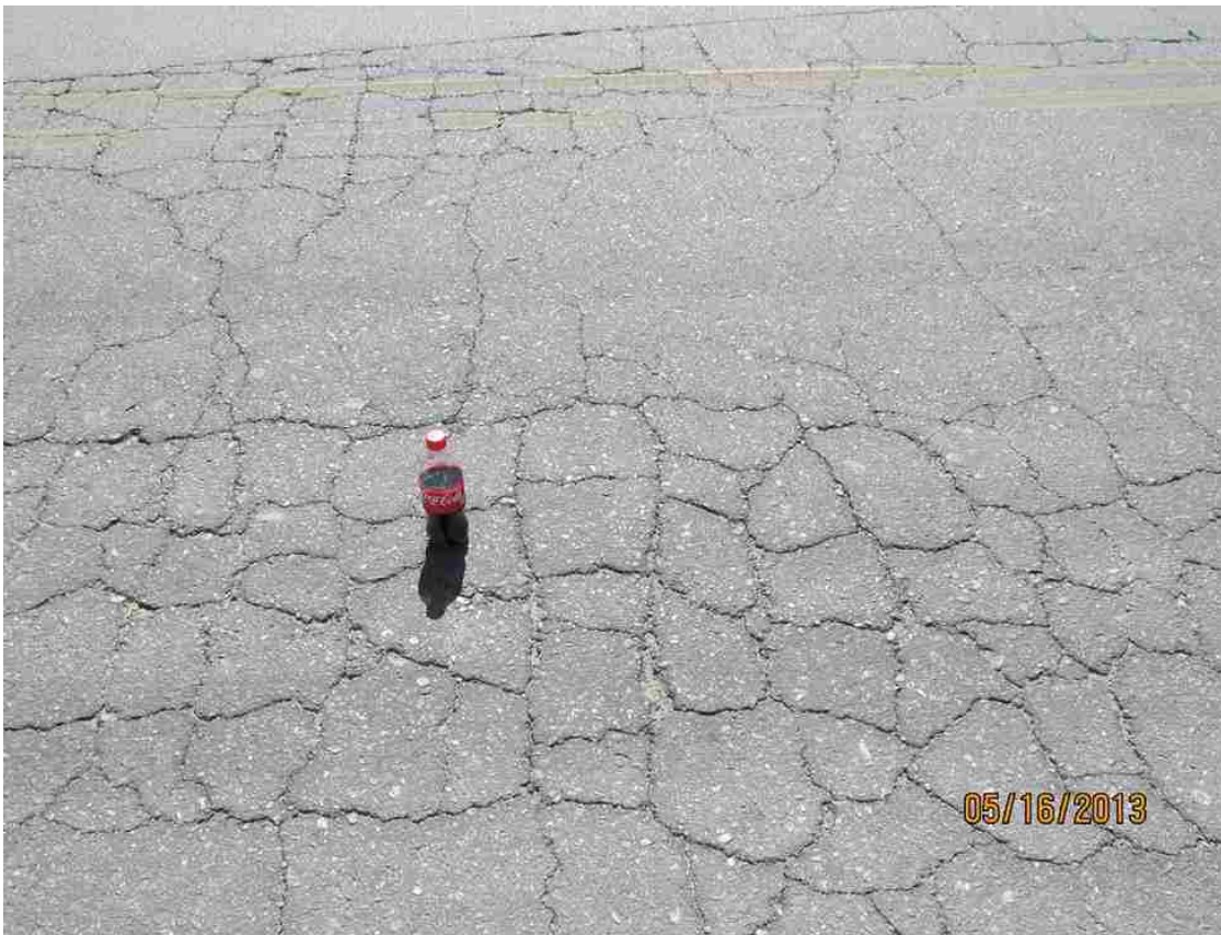
Figure 3. Pavement alligator cracking
