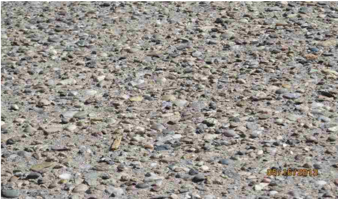
Figure 1. Raveling and weathering of flexible pavement
