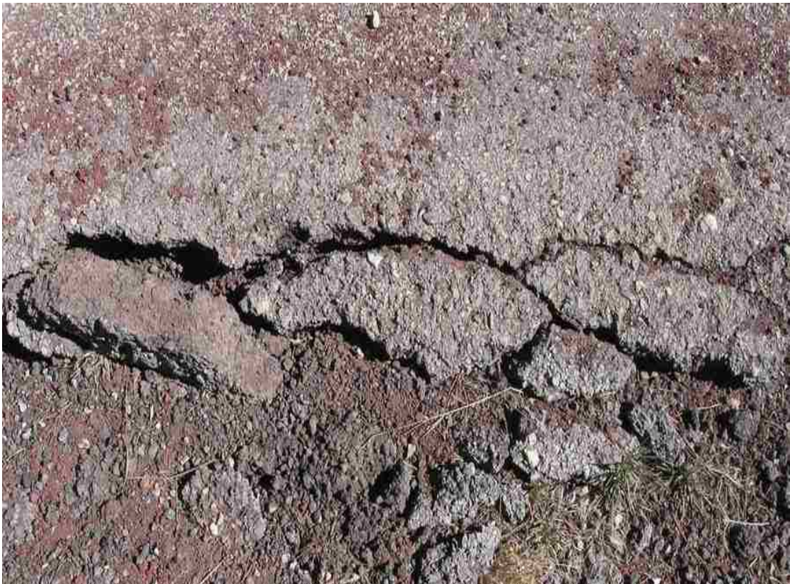
Figure 5. Edge cracking of flexible pavement
