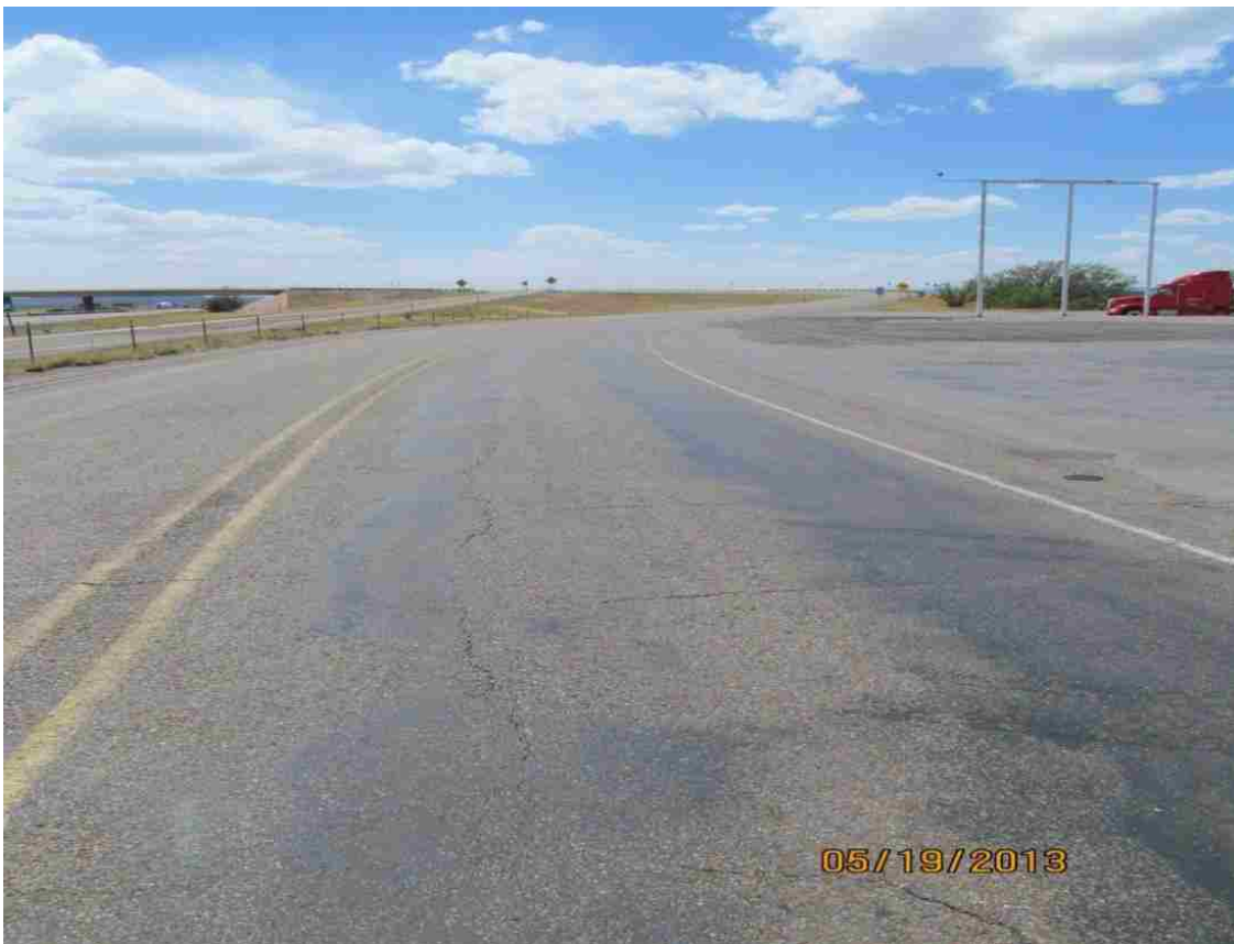
Figure 2. Pavement asphalt bleeding
