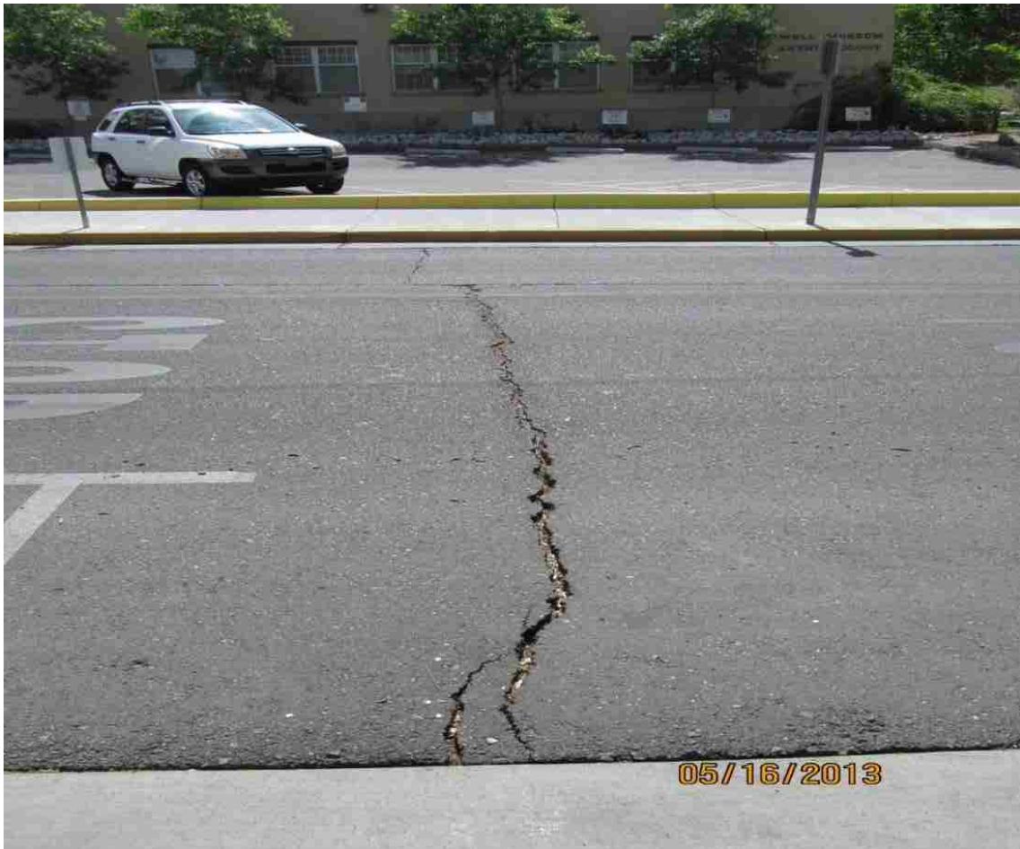
Figure 4. Transverse pavement cracking
