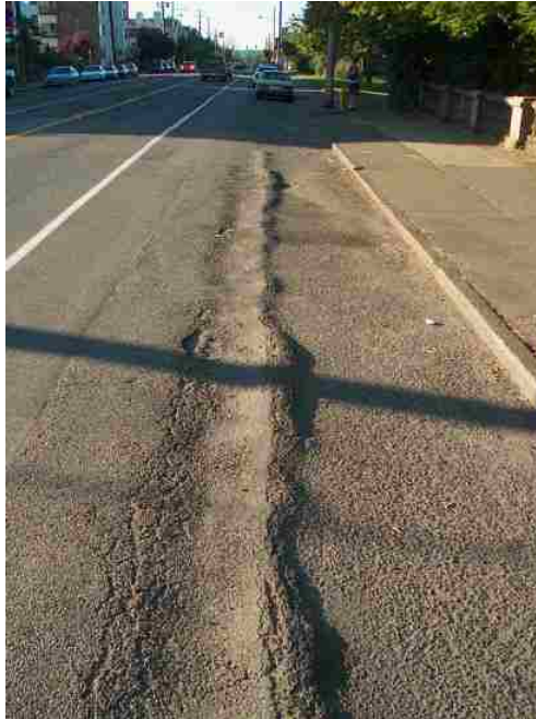
Figure 2.1 Permanent deformation distress
