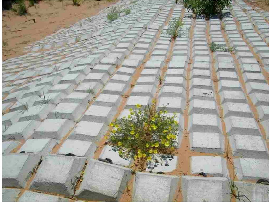
Figure 8: Articulating concrete mat at one of Submar’s testing sites in Southeast New Mexico. Photo courtesy of Submar.
