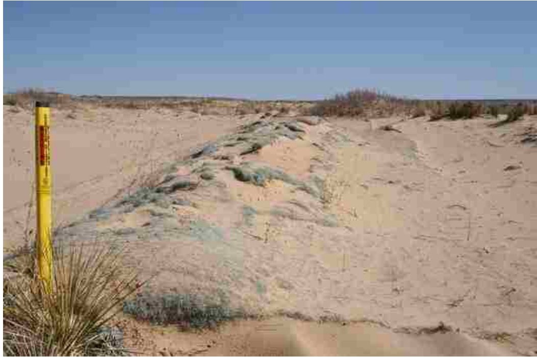
Figure 10: One year old geotextile repair, placed over sand mounded on top of exposed pipeline. Geotextile is already being torn away from repair. Photo: Knutt Peterson
