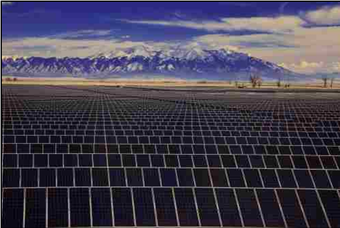
Figure 1. The 8.22 MW SunEdison/Xcel Energy Photovoltaic (PV) Power Plant Outside of Alamosa, CO.
