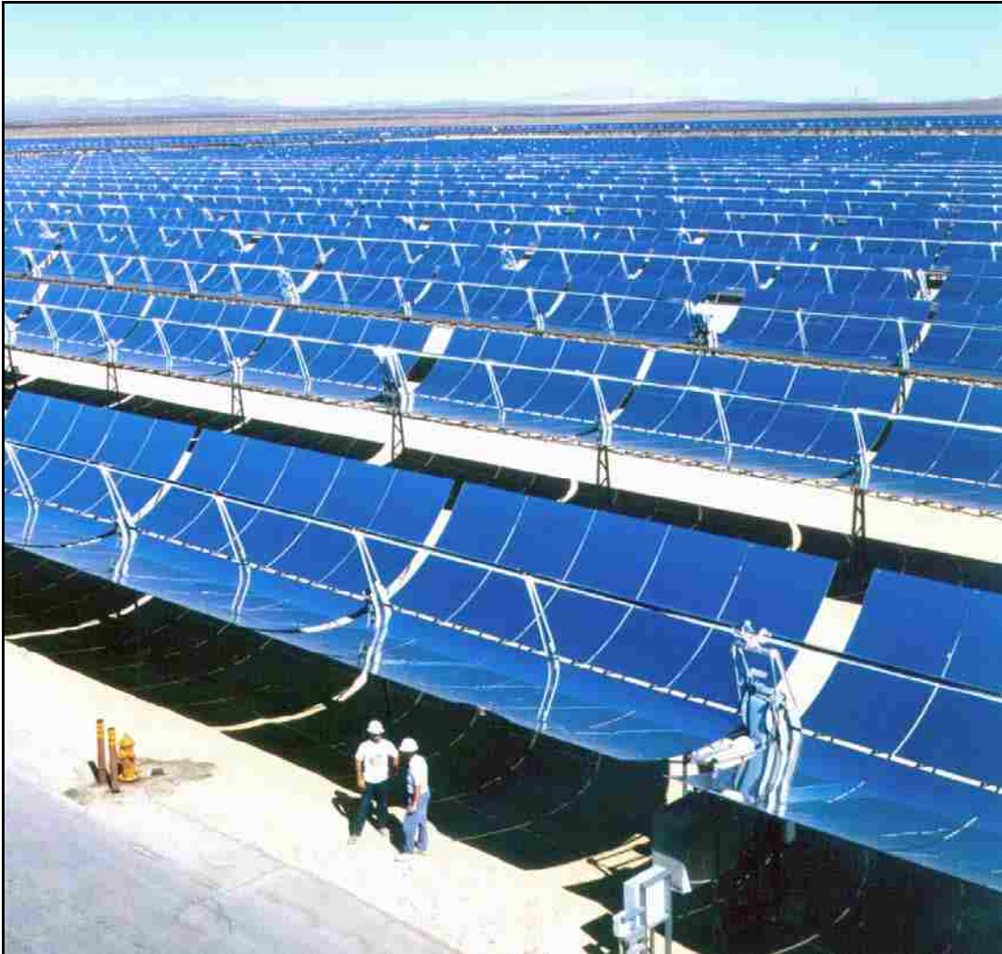
Figure 2. Parabolic Trough Mirrors at the SEGS IV CSP Facility in Kramer Junction, CA.
