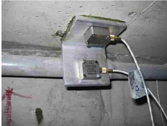
Figure 2-3. Accelerometers installed on a bridge to measure bridge displacements (Sheppard 2010)
