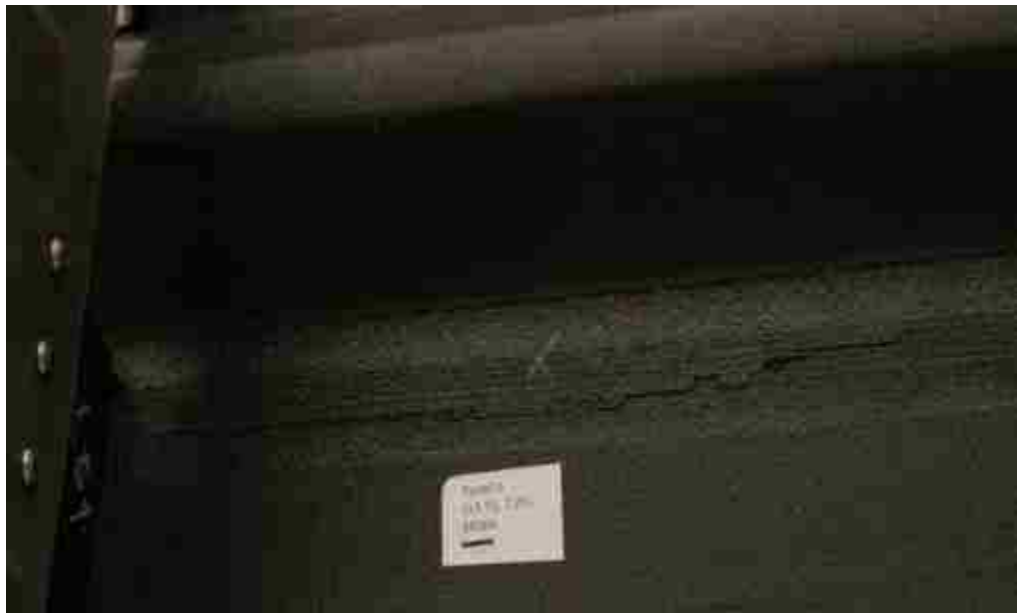
Figure 4-15: Stringer Flange Delamination Detectable from Backside of Panel A
