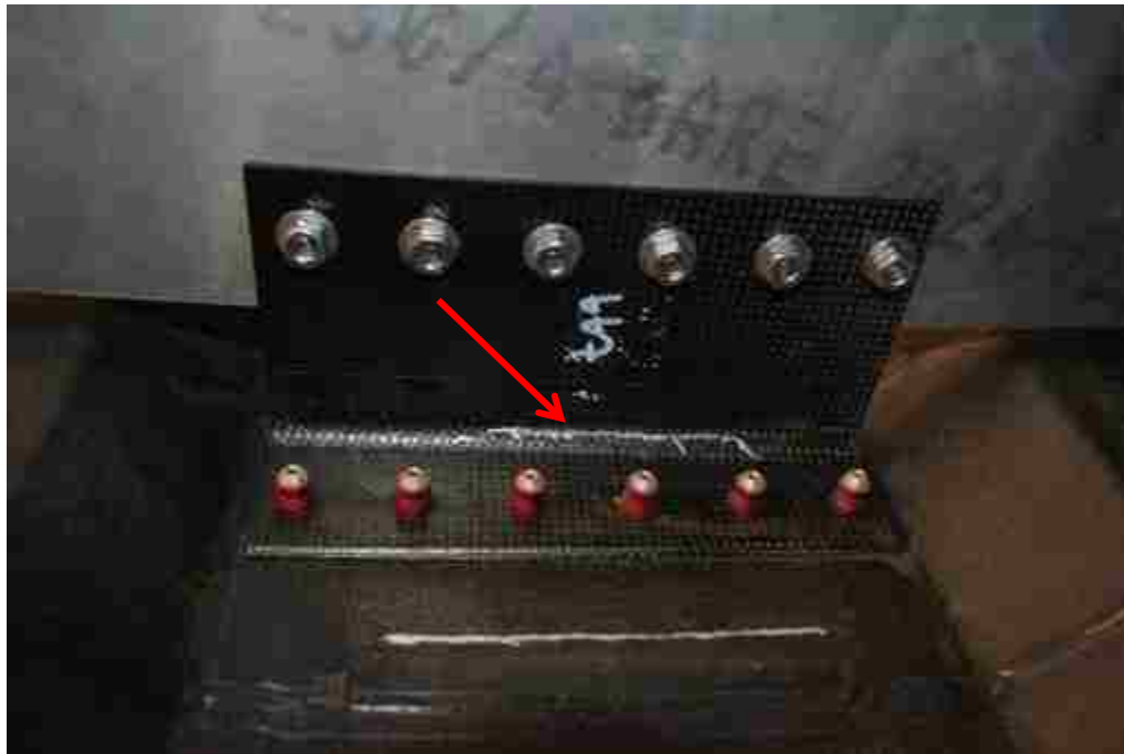
Figure 4-16: Crack on Shear Tie Bend Radius Not Detectable Using NDI from Front Side of Panel
