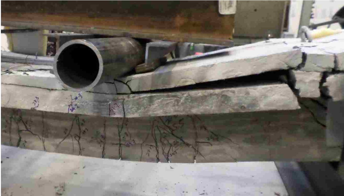
Figure 4.35: Debonding of UHPC overlay in Beam-UF at support area
