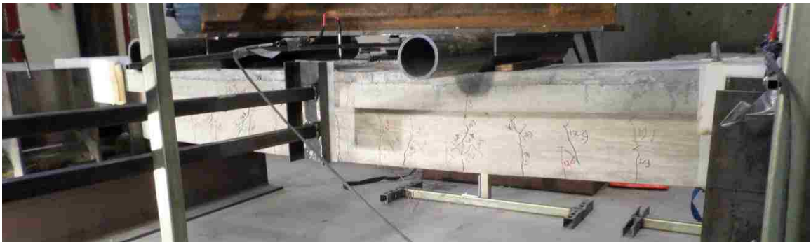
Figure 4.45: Cracks propagated in Beam-MUF at early loading
