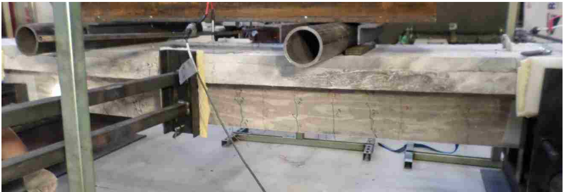
Figure 4.33: Vertical cracks in Beam-UF
