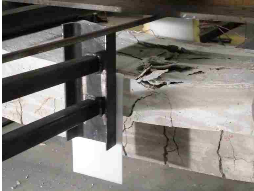
Figure 4.13: Crushing of Concrete at Beam-C
