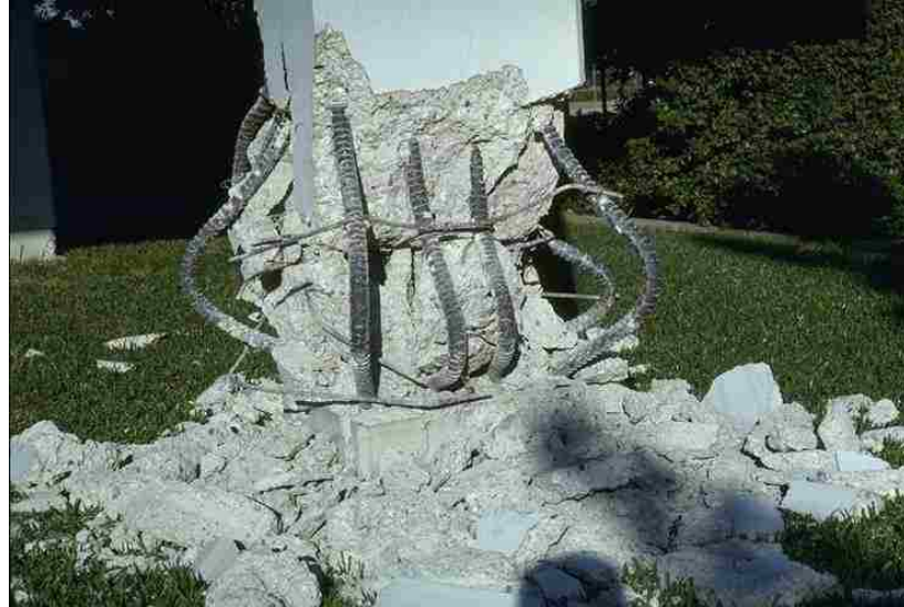
Figure 1.1 – Failure mechanism at the bottom of a concrete column subject to earthquake loading (from [Jennings 1971]).
