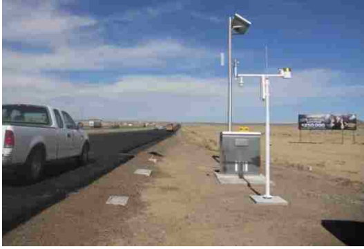
Figure 23. Installed weather station
