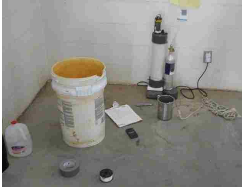
Figure 34 Sampling Set-Up in PTF Blower Building
