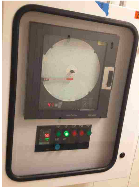
Figure 3.4.6.1 Control system of the freezer room
