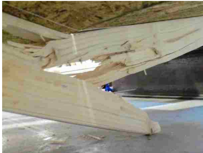
Figure 3.11 Failure of T-beam at a knot close to the gap in the OSB.
