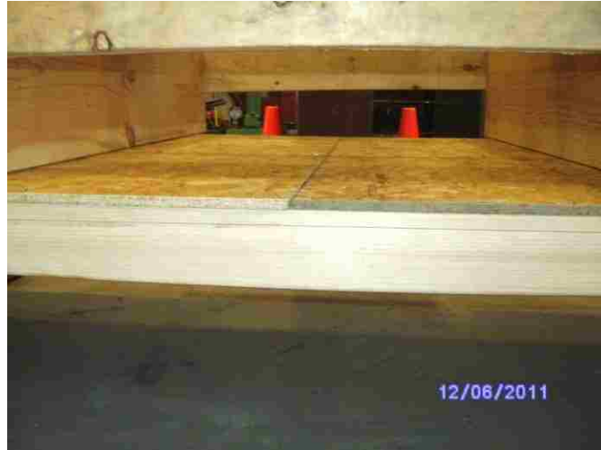
Figure 3.4 Gap at midspan in OSB sheathing.
