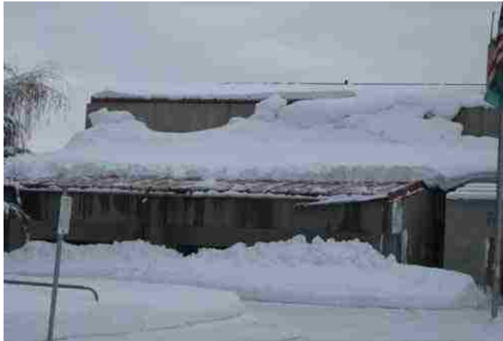
Figure 6.1 Snow sliding. From study of structural failures associated with the winter 2008-2009 snow event in the Spokane/Coeur d'Alene area [SEAW, 2009].
