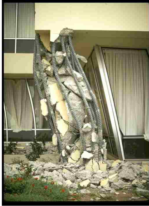
Figure 1.2 - Damaged column at Olive View Hospital, from [Steinbrugge 1992]
